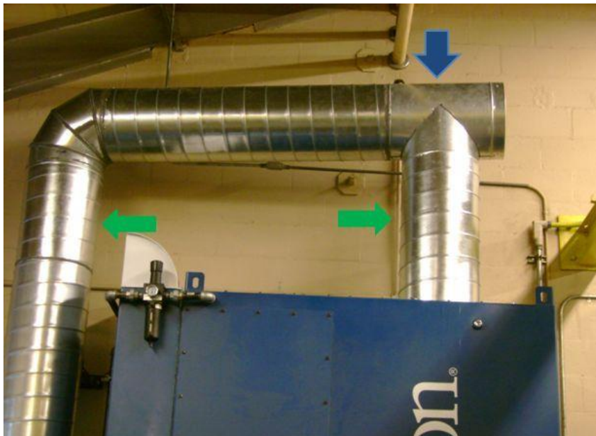
Figure 7. Duct routing to plasma table after project.
