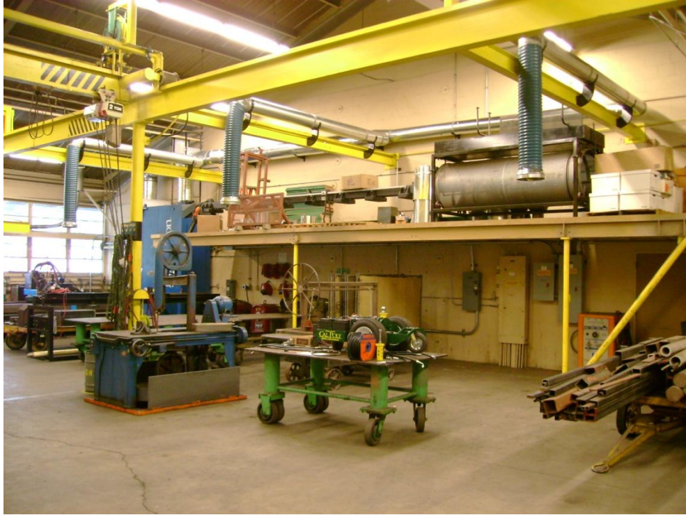
Figure 18. Another view of completed system.
