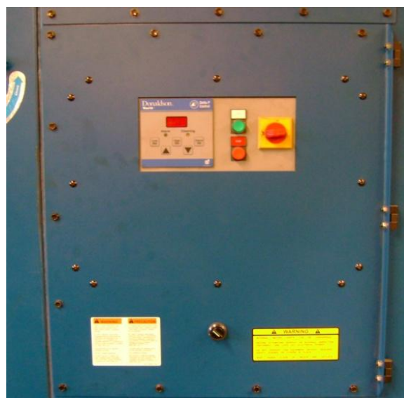
Figure 12. TG8 control panel and air control selection switch.
