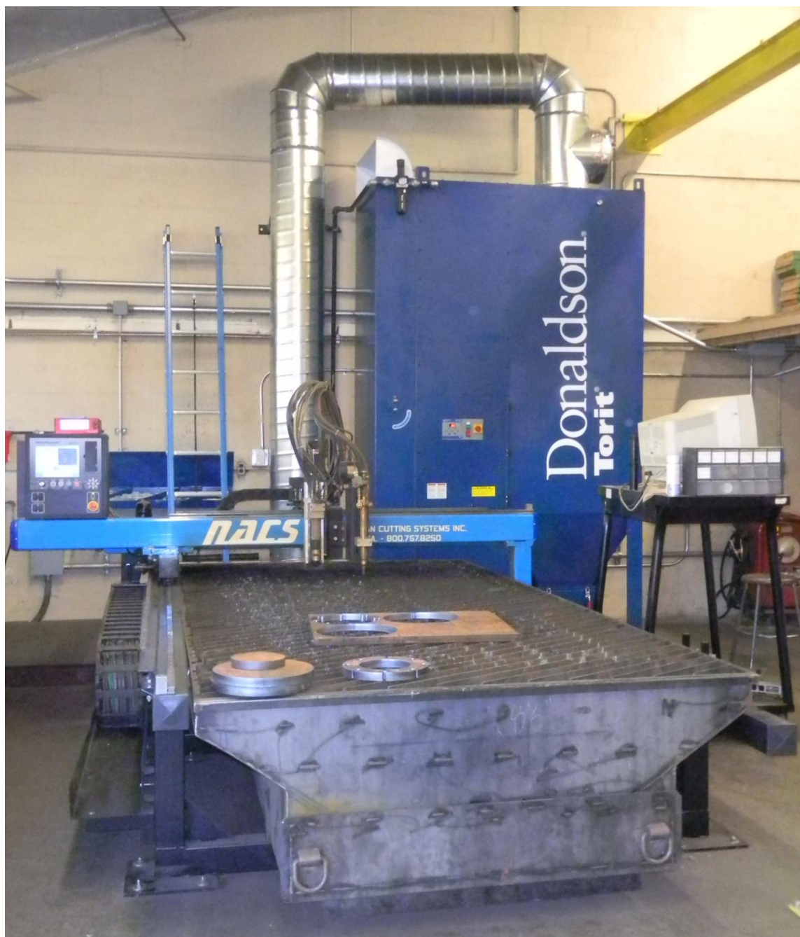
Figure 1. Original installation of Donaldson Torit Powercore TG8 dust collector in BRAE Lab #6.
