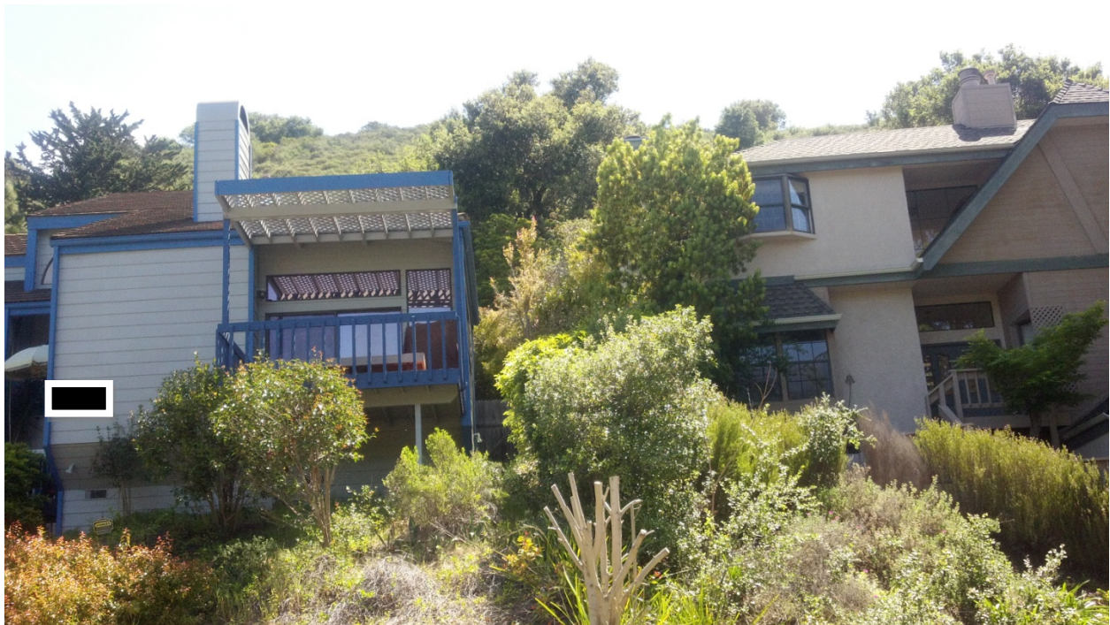
Figure 22. Wooden deck with vegetation underneath and tree against a home
