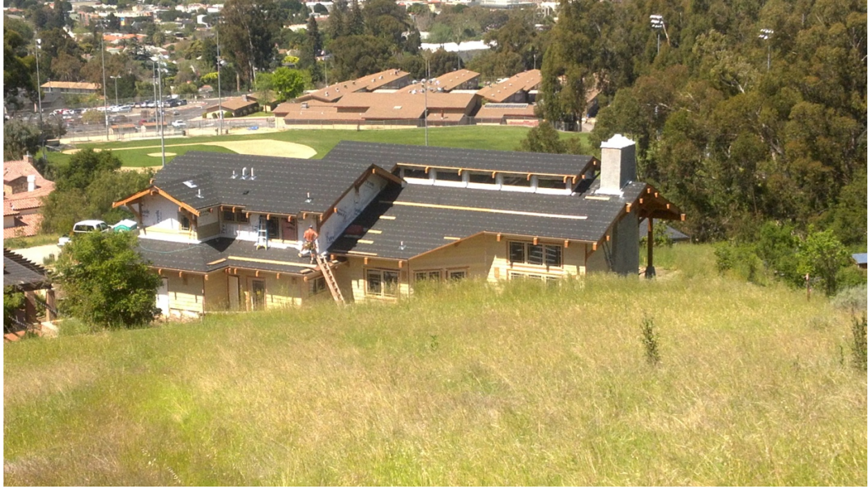
Figure 26. Home construction with dry grass adjacent to the site
