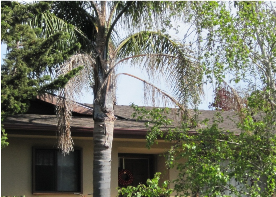
Figure 40. Un-pruned palm tree overhanging wooden roof
