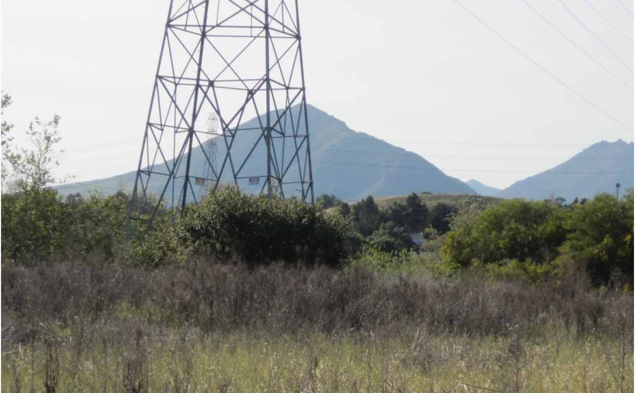
Figure 34. Vegetation growing underneath an up to transmission lines
