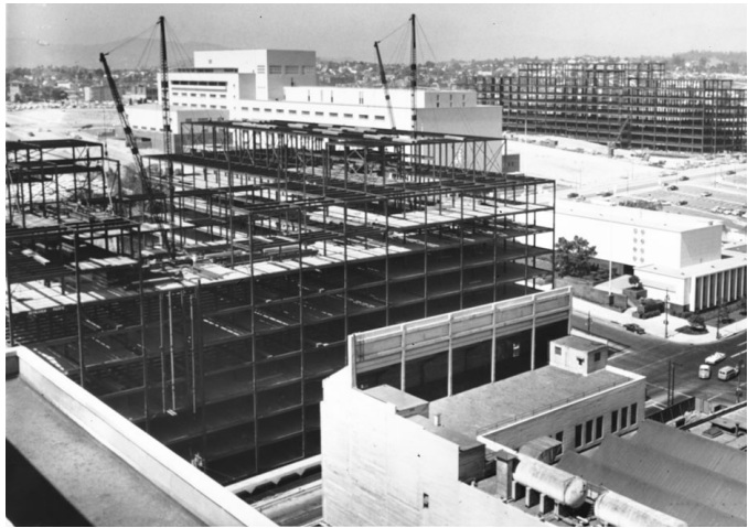
Figure 5.16. (Left) View looking northwest over the intersection of 1st and Broadway showing the construction of State Office Building No. 2 (foreground) and the LA County Hall of Administration (background), September 11, 1958 ( The Examiner )
