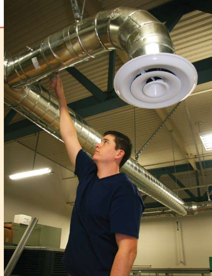
Heating, Ventilation, Air Conditioning and Refrigeration student Jeff Wong works with some of the new equipment in the refurbished Critchfield Lab.
