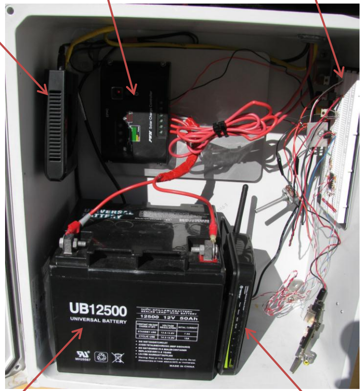
Figure 30: Interior of Battery Box
