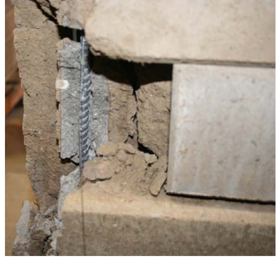
Figure 6-38: Unconfined rebar in tension during the push excursion of Cycle 24.
