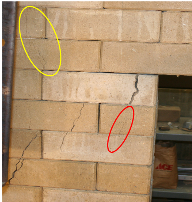
Figure 6-50: New cracks observed in W6 during Cycles 9 and 10
