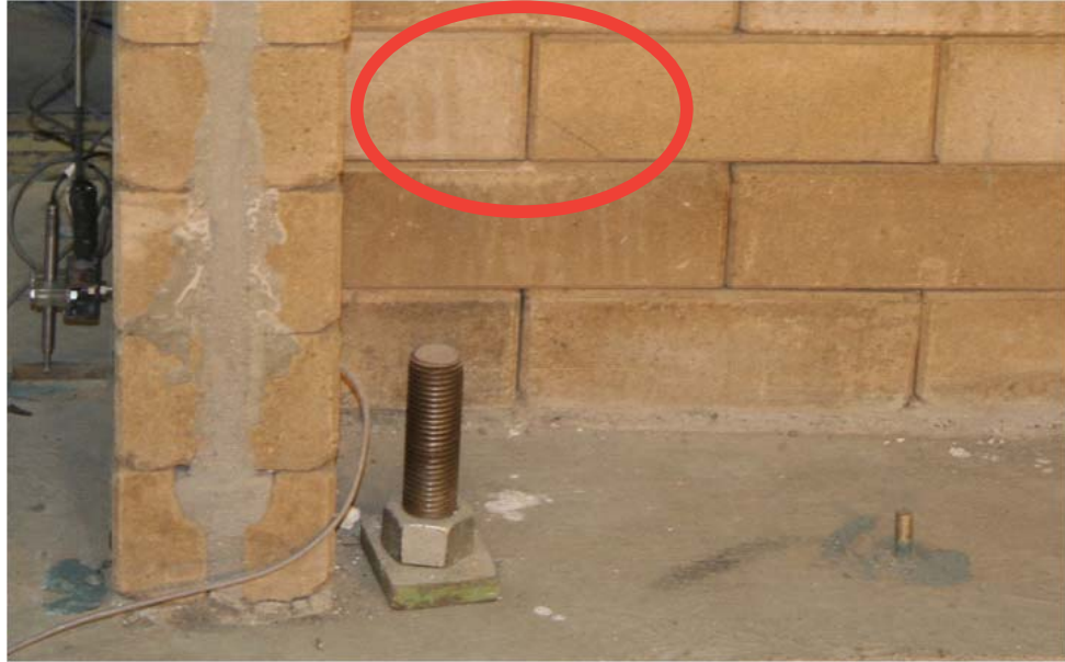
Figure 6-26: Crack in W5 at zero displacement
