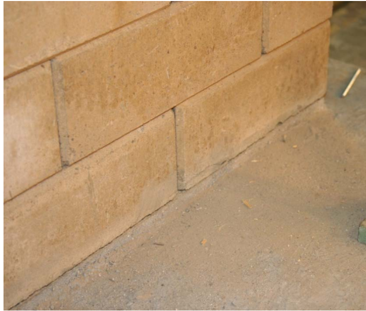
Figure 6-5: Cracking at the base of W4 during Cycle 10
