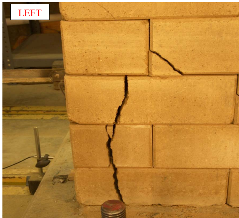
Figure 6-13: Toe cracking of W4 in Cycle 24
