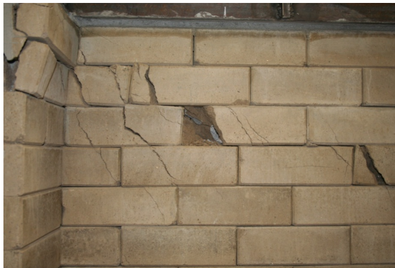
Figure 6-20: Shear Failure of the web and flange.
