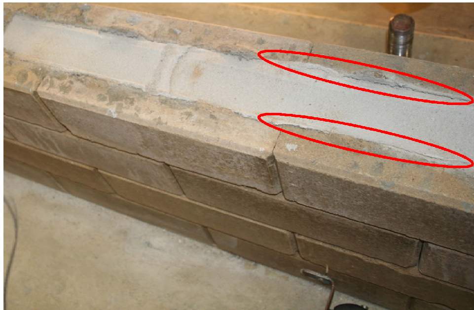
Figure 6-47: W6 cracking around the sill of the windows following Cycle 14
