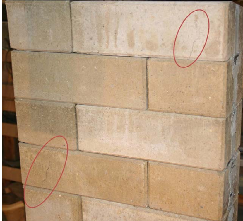
Figure 6-48: W6 diagonal cracking observed in the left pier after Cycle 16
