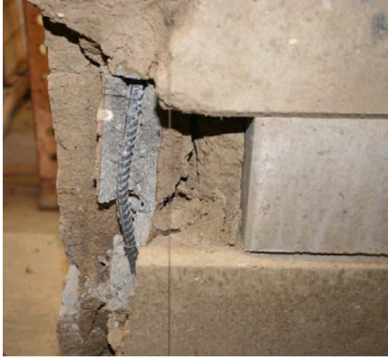
Figure 6-37: Buckling of unconfined rebar subjected to compressive force during pull excursion of Cycle 24.
