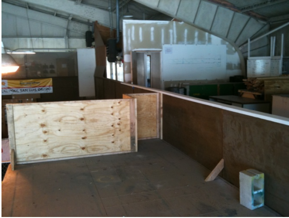
Figure 20 - Cleared Balcony. Some railing left over for potential of new railing project
