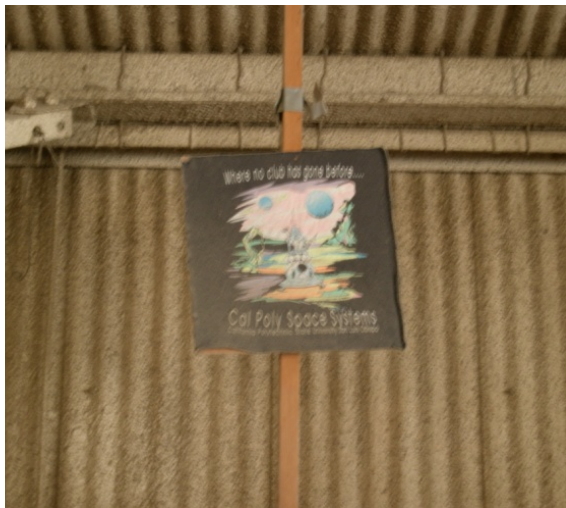
Figure 3 - Asbestos covers the workspace CPSS must use
