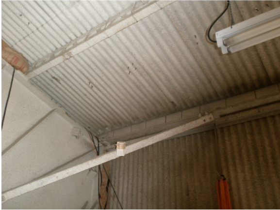
Figure 21 - Asbestos covered room intended for enclosure
