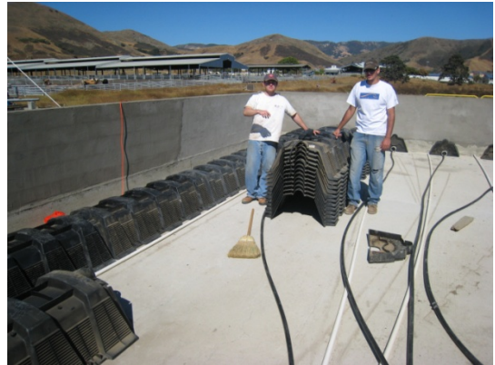
Figure C.4. Installation of Biodiffuser leach field chambers. Black and white pipes will run along floor and connect to aerator manifold. Black pipes lie underneath chambers, white pipes lie between chambers.
