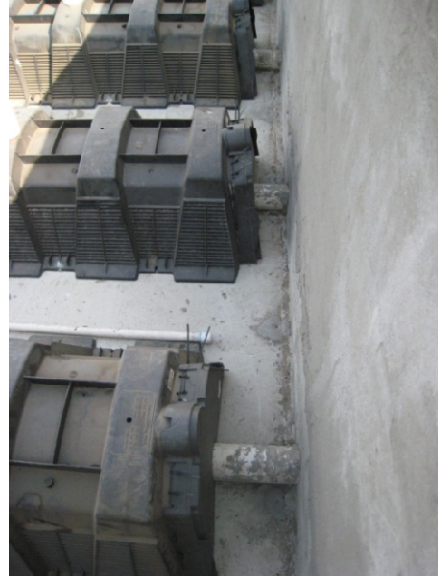
Figure C.11. Pipe penetrations connecting leach field chambers to outside of basins. Extend approximately 30-cm into chamber and provide conduit for sludge removal.
