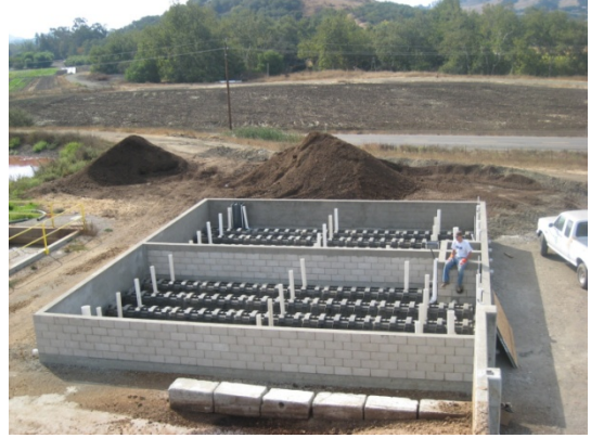
Figure C.7. View of leach field chamber network from solid chamber network from solid separation screen.
