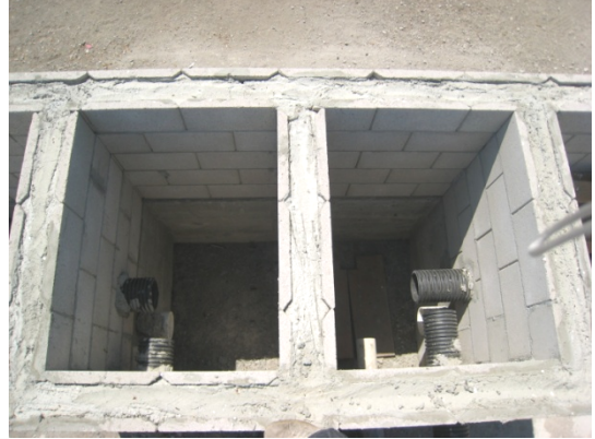
Figure C.3. Sumps with pipe penetrations. Black perforated pipes assist in draining basins, white pipe in right sump is connected to weir box in Basin 2.
