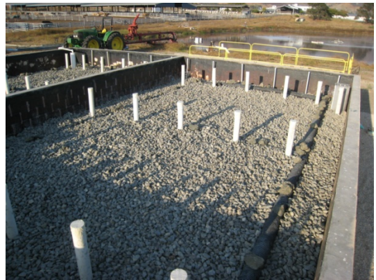
Figure C.12. Basin 2 after installation of two rock layers. Black perforated pipe network, installed to assist drainage.
