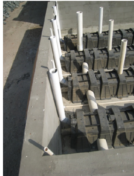
Figure C.8. Leach field chamber network along western wall. Large white pipes along wall house black aeration tubes running up from underneath chambers. Small white pipes along wall are aeration pipes running between chambers. Large white pipe sections connecting chambers help drain basin.
