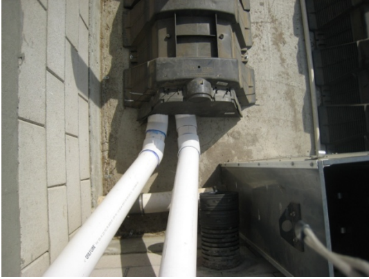
Figure C.9. Weir box in south tank near sump. Controls water level in north tank. Pipe on floor connects weir box to Basin 1.
