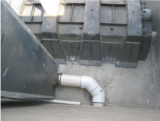
Figure C.10. Effluent pipe connecting to effluent weir.
