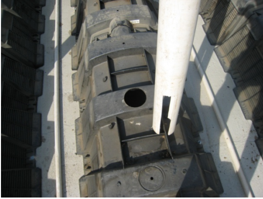
Figure C.5. Installation of standpipes into leach field chambers. Slots in pipe leave room for black aeration pipes lying on basin floor.
