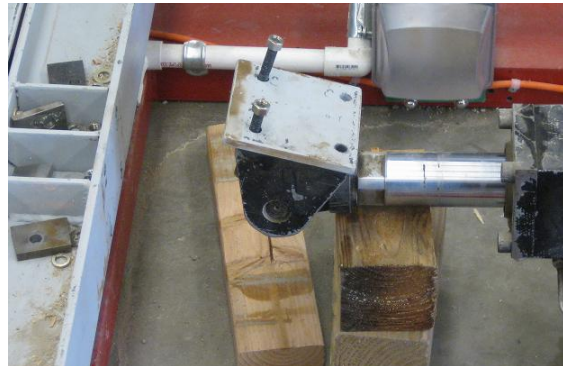
Figure P - Disconnected hydraulic pump
