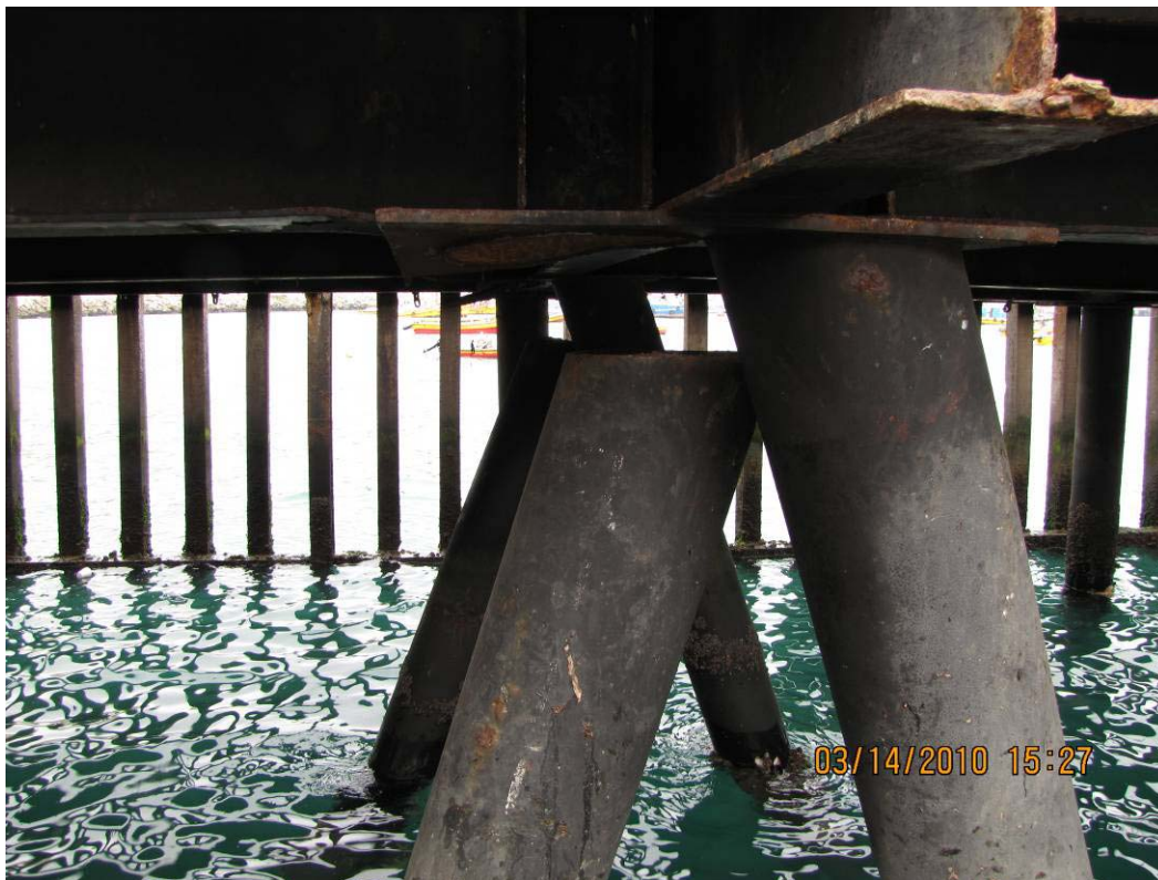
Figure 8.36. Failure of head connection between wharf and raked piles in San Antonio Port (S33.5817°, W71.6154°; 1527 hrs, 03/14/2010).
