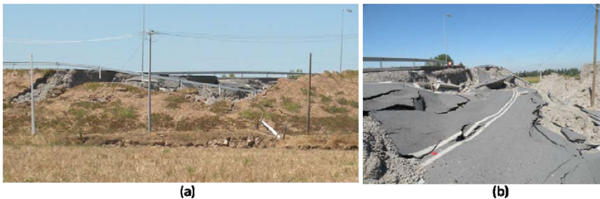
Figure 9.58. Curved overpass embankment failure 13 km North of Parral (a) Translational 3-D slide failure, (S36.0343 W71.7568; 1405 hrs on 3/11/2010) and (b) Failed outside of the curved embankment (S36.0347 W71.7558; 1409 hrs on 3/11/2010)
