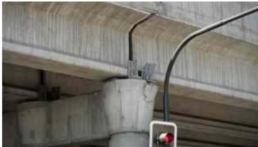
Figure 5.7. Paso Lo Boza (S33.3865° W70.7601°). Minor structural damage of shear keys (Source: Dr. Roberto Leon, personal communication).
