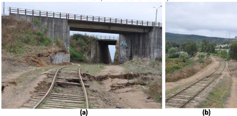
Figure 9.56. Lota (a) Slab and girder-type overpasses at northern end of road embankment failure area, showing railroad and supporting ground settlement. View looking west. (S37.0729°, W73.1469°; 1150 hrs on 3/16/2010), (b) Ground failure below elevated railroad east of road embankment failure. (image looking east; S37.0727°, W73.1471°; 1150 hrs on 3/16/2010)
