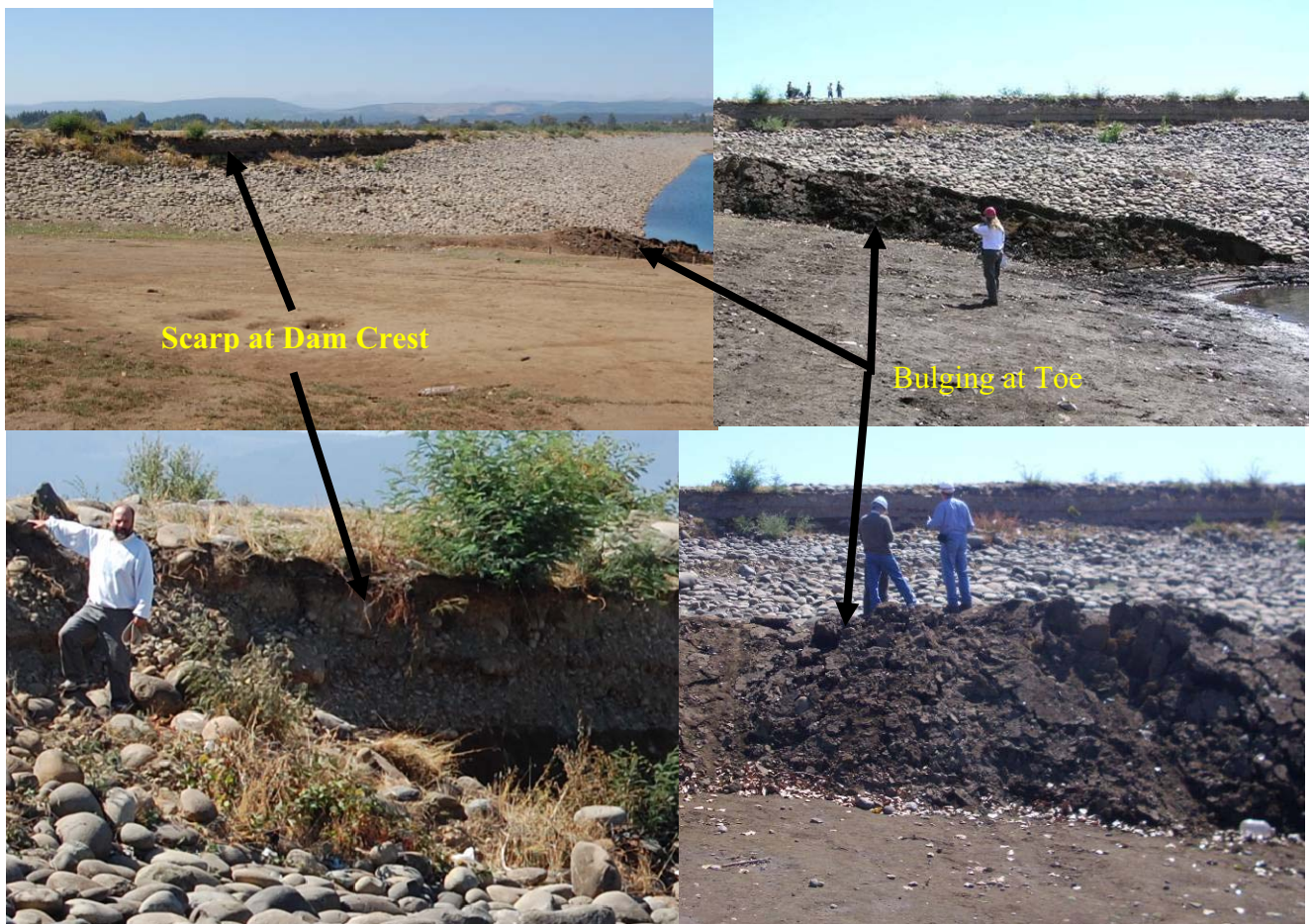
Figure 11.2. March 10, 2010. Slump of the upstream face of Coihueco Dam near the left abutment (S36.637166°, W71.797530°)
