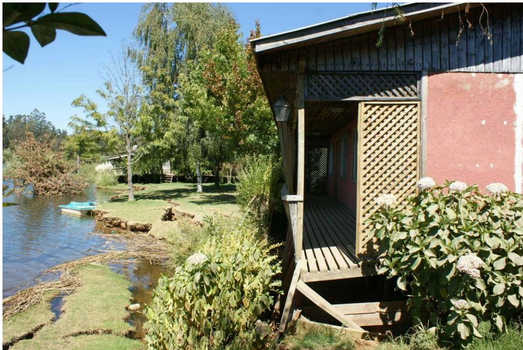
Figure 14.13. Lago Vichuquen. Lateral spreading has affected much of the ground underlying a small lakeside cabana hotel. Some shore side piers of the cabanas were submerged and there was evidence of structural damage as well. (S34.796345°, W72.07885°; 12:58 hours on 3/15/2010)
