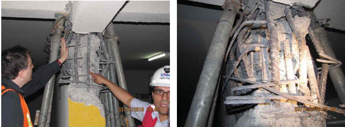
Figure 5.26. Site DA027 (S 33.020074° W 71.544055°, 1945 hrs on 03/15/2010). Heavily damaged 20-story building, lack of confinement at beam-column joints.
