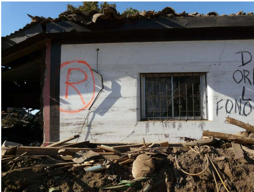
Figure 13.25. Watermarks on damaged buildings in Constitución indicate tsunami flow depths reached at least 2 m along the waterfront on Calle Blanco (S35.336 W72.403, 1757 hrs on 03/15/2010).
