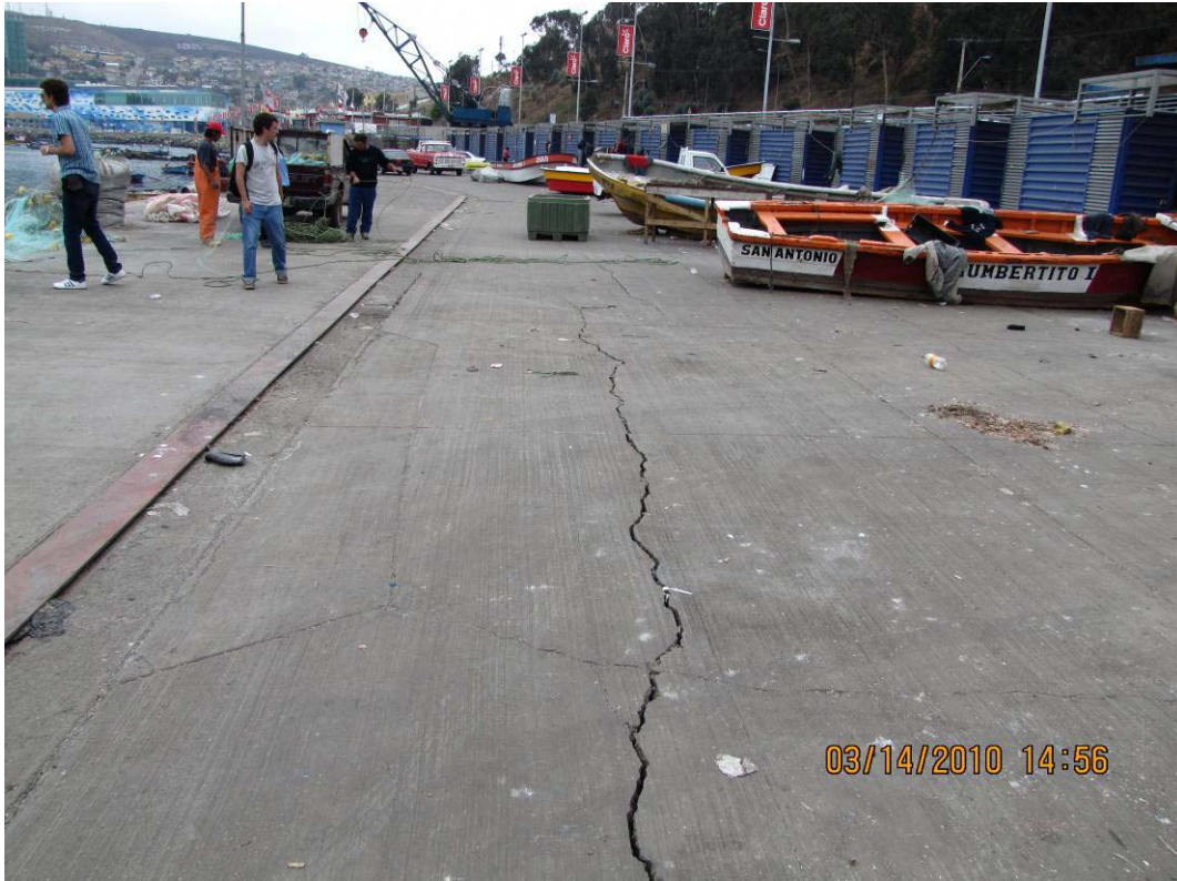
Figure 8.31. Cracks on asphalt pavement behind quay wall in San Antonio Port (S33.5870°, W71.6132°; 1456 hrs, 03/14/2010).
