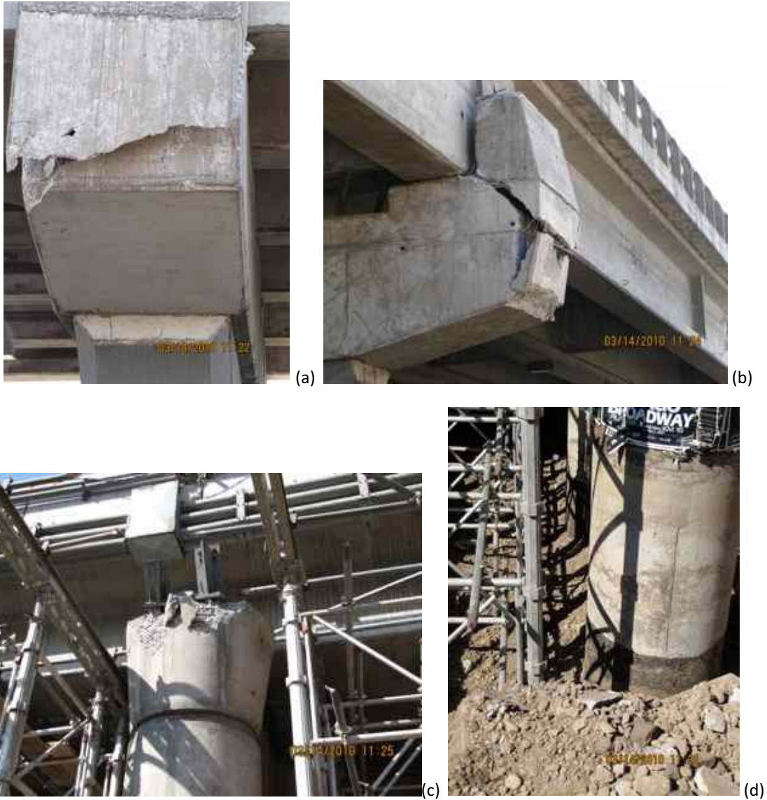
Figure 5.5. Paso San Martin (S33.3660° W70.6891°, 1122 hrs on 03/14/2010). Shear key failure and longitudinal, transverse deck displacement.
