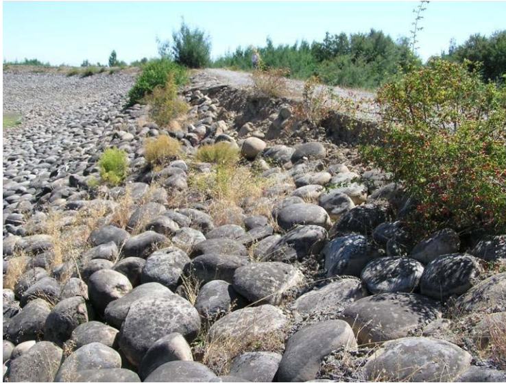
Figure 11.4. March 10, 2010. Small Area of Upstream Crest Slumping on Coihueuco Dam (S36.636902°, W71.788897°)
