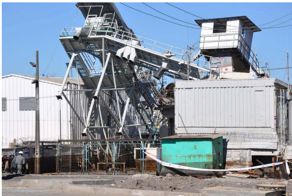
Figure 8.27. Damage to structures neighboring the fish packaging facility (S36.7267°, W73.1282°; 1200 hrs, 03/15/2010). Note the scum level at the base of the structure of approximately 1-2 m evidence of the water rise.
