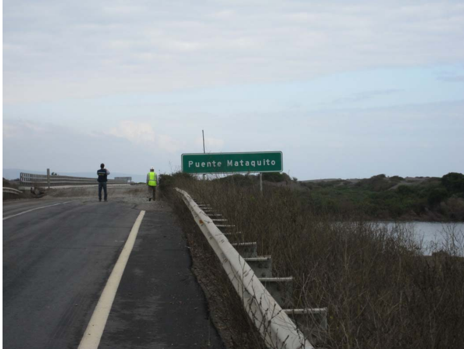
Figure 15.66 Settlement of the north abutment of the bridge, 70 cm offset at the bridge deck, Puente Mataquito, 35.050712°S, 72.162258°W, April 16, 2010.
