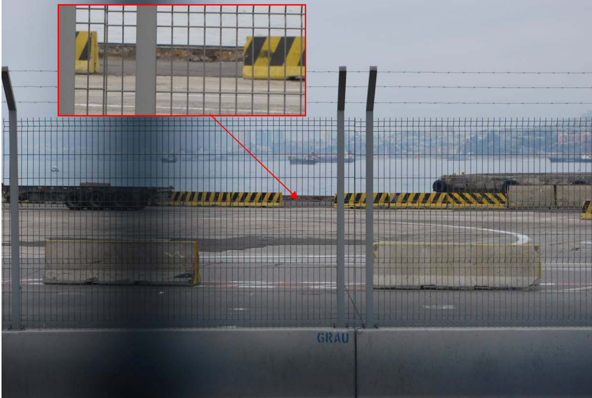
Figure 8.19. Settlement in backfill behind the quay wall at commercial dock of Valparaiso port (S33.034°, W71.627°; 1620 hrs, 03/15/2010).
