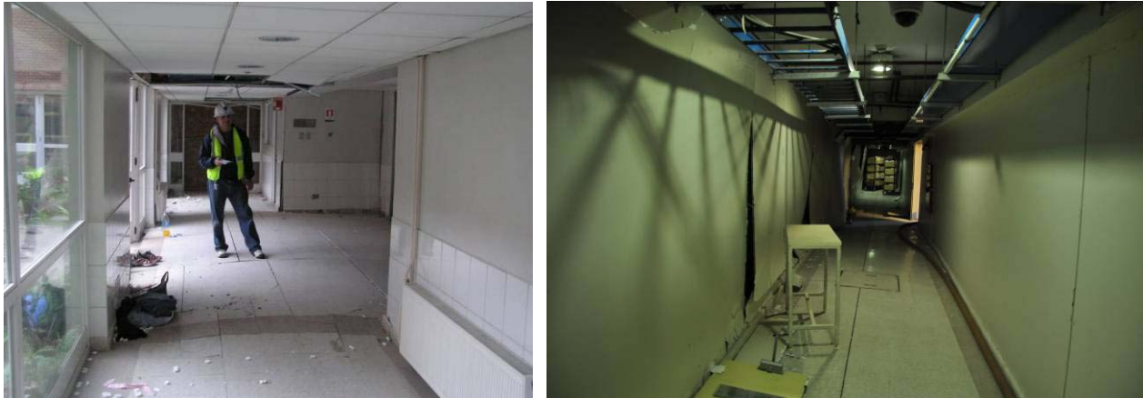
Figure 7.9. Distortion of the slab-on-grade: (a) floor bulging in front of elevator shaft in Wing 1C (S37.47345°, W73.34835°), and (b) floor distortion in eastern hallway of Wing 1B (S37.4733°, W73.3478°).
