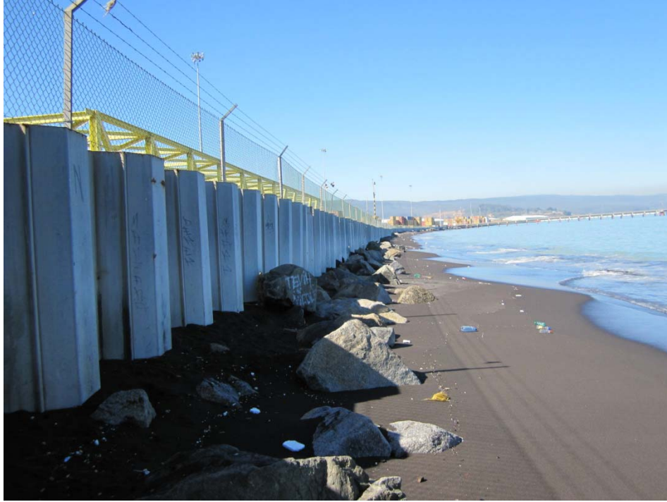
Figure 15.78 Seaside view of the sheet pile wall that experienced lateral spreading, Port Coronel, April 14, 2010 (37.028874°S, 73.149768°W).
