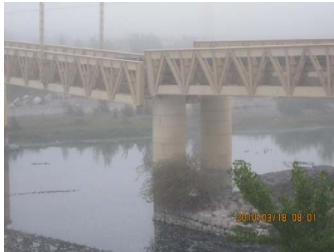
Figure 9.63. Unseated railway bridge span near Longavi from excessive transverse movement (S36.004136, W71.726193, 0801 hrs on 3/18/2010)
