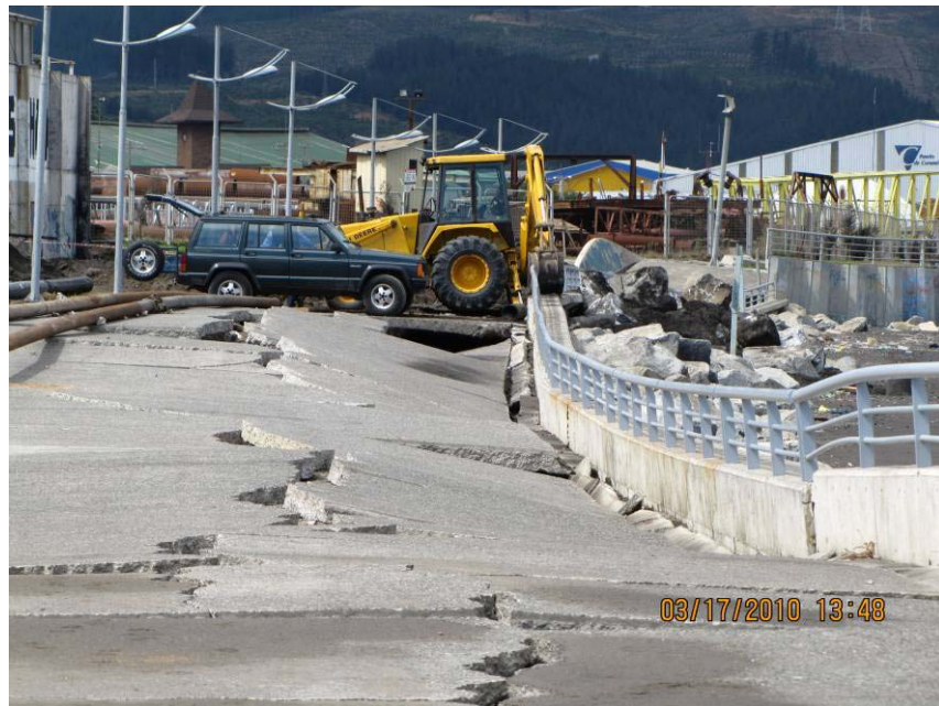
Figure 8.10. Photograph of lateral spreading which destroyed pavement and cracked walls at the fishermen's Port of Coronel (S37.0247°, W73.1550°; 1348 hrs, 03/17/2010).
