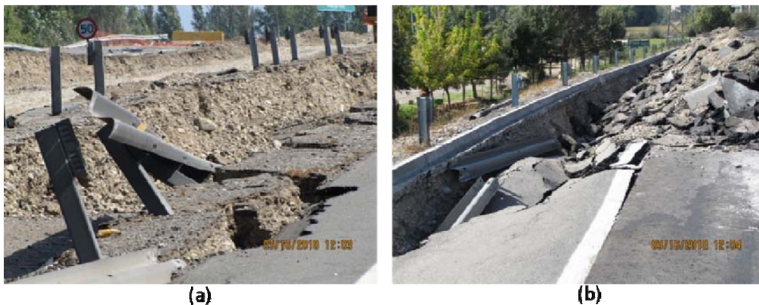
Figure 9.60. Highway 5 failure near Paine; (a)shoulder settlement due to poorly compacted soil (S33.864897° W70.742222° 1203 hrs on 3/16/2010), and (b) road failure due to poorly compacted soil (S33.864897° W70.742222°; 1204 hrs on 03/16/2010)
