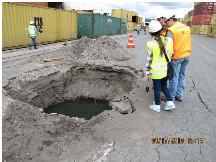
Figure 8.5. Development of sinkholes (2.2 m deep, 3.5 m diameter) as a result of crack (gap) in pipe (S37.0339°, W73.1467°; 1513 hrs, 03/17/2010).
