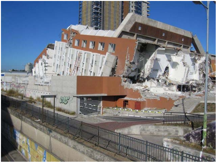
Figure 15.57. Collapsed 14 story building, Concepcion (36.82779S, 73.060777W)
