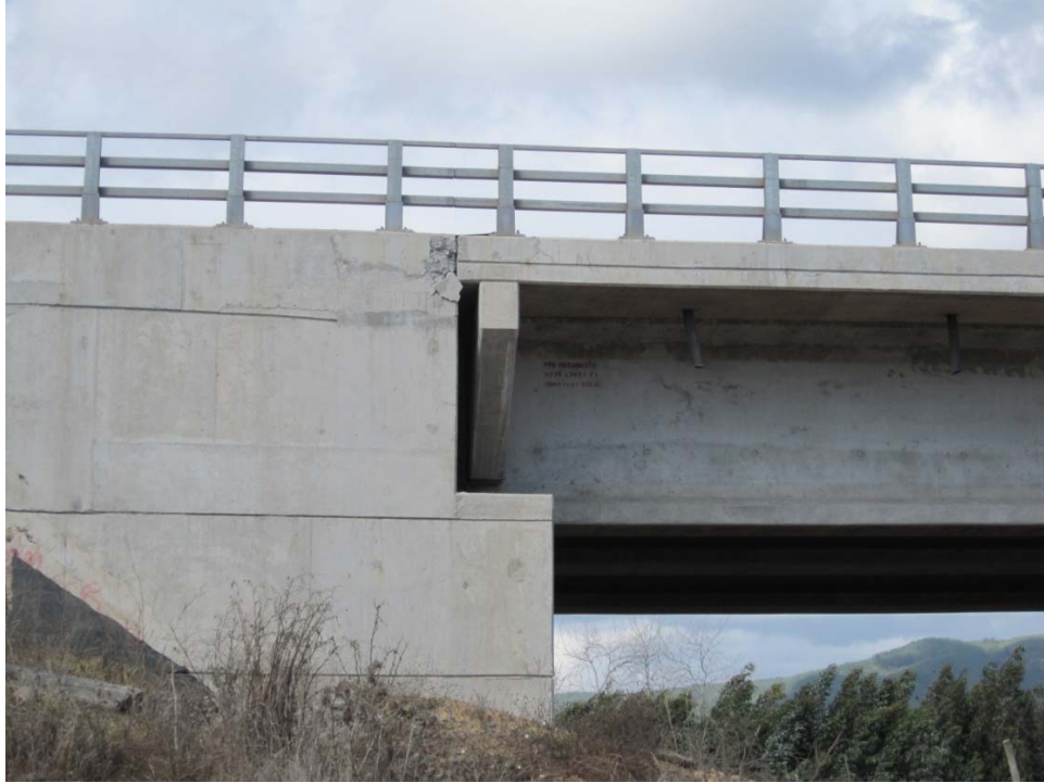
Figure 15.70 North abutment shoved into bridge deck due to lateral spreading, Puente Mataquito, 35.050712°S, 72.162258°W, April 16, 2010.
