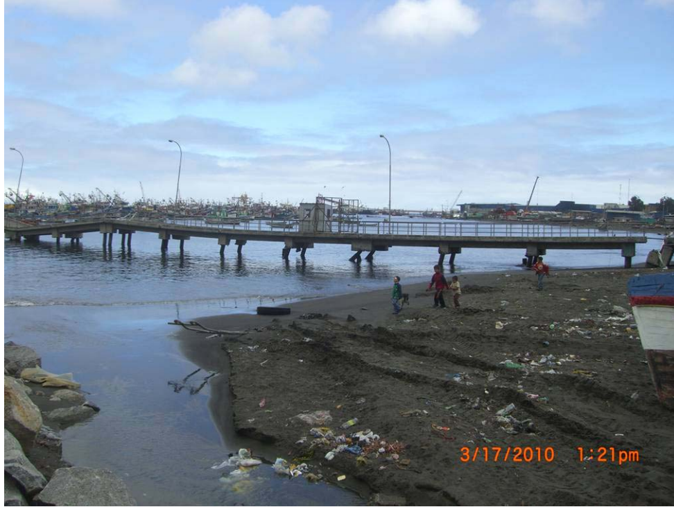
Figure 8.12. Damage to pile supported pier at small fishermen's Port of Coronel due to lateral spreading (S37.024319°, W73.156210°; 1321 hrs, 03/17/2010).
