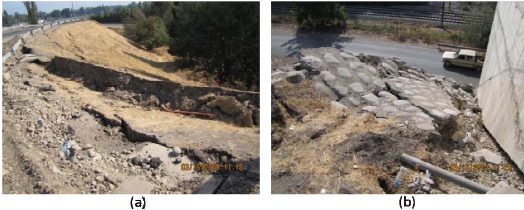
Figure 9.59. Highway 5 crossing near Paine; (a)View of bridge approach from East (S33.854592° W70.747687°; 1118 hrs on 3/16/2010); (b) View of damaged bridge abutment (S33.854211° W70.747784°; 1120 hrs on 3/16/2010)
