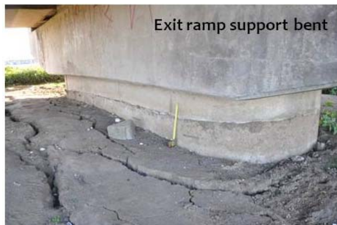
Figure 9.7. Ground settlement surrounding an exit ramp support bent at the Llacolén bridge in Concepción (S36.830380°, W73.067541°, 1901 hrs. on 3/14/2010).
