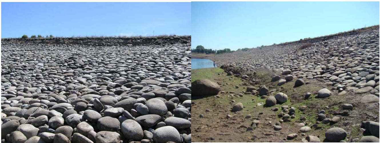
Figure 11.3. March 10, 2010. Slumping at Coihueco Dam Crest and Bulging at Dam Toe. (S36.636508°, W71.792505°)
