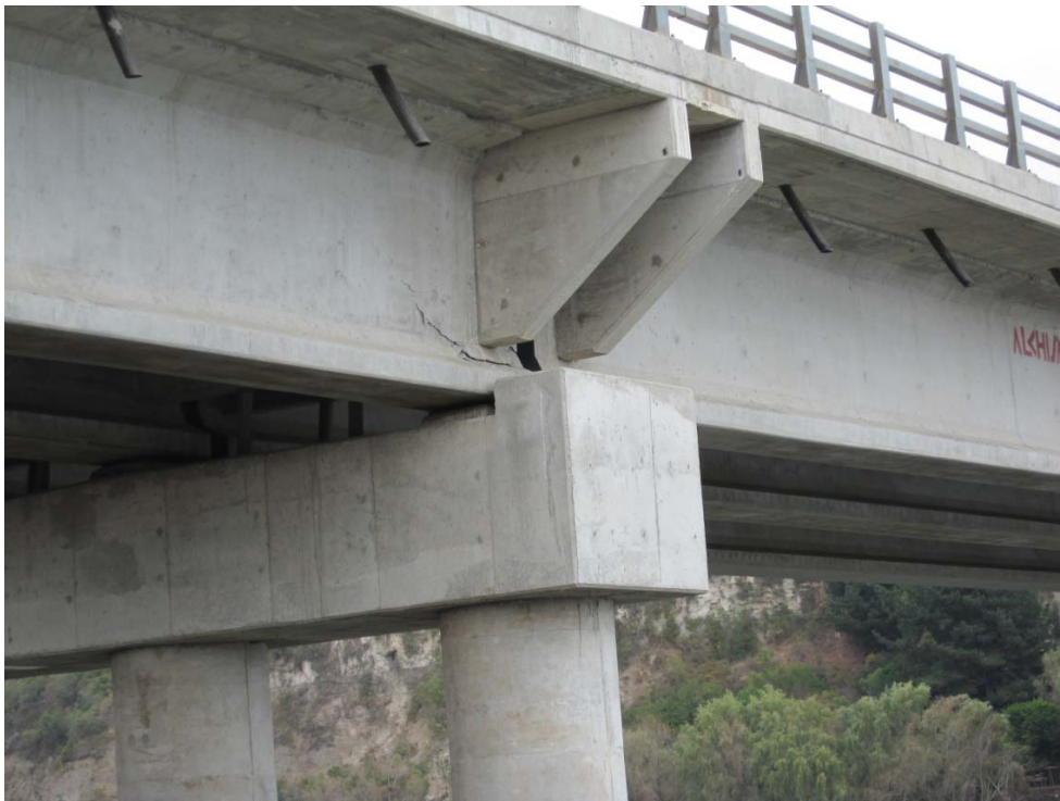
Figure 15.71 Shearing of bridge girder, North abutment of bridge, Puente Mataquito, 35.050712°S, 72.162258°W, April 16, 2010.
