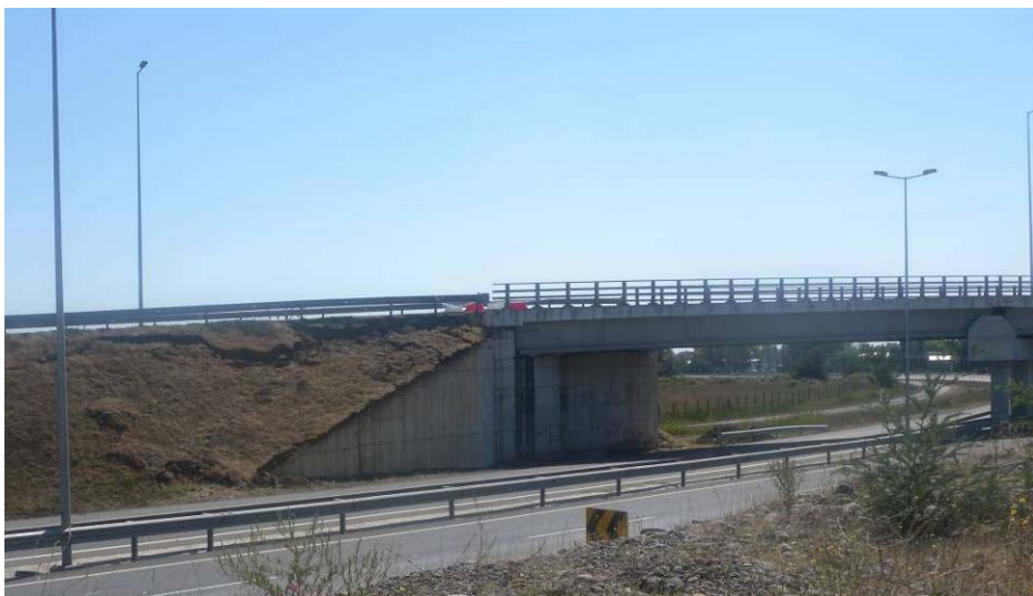
Figure 12.6. Surficial sloughing on a bridge approach embankment, with the abutment showing no evidence of damage, Route 5, north of Chillan.
