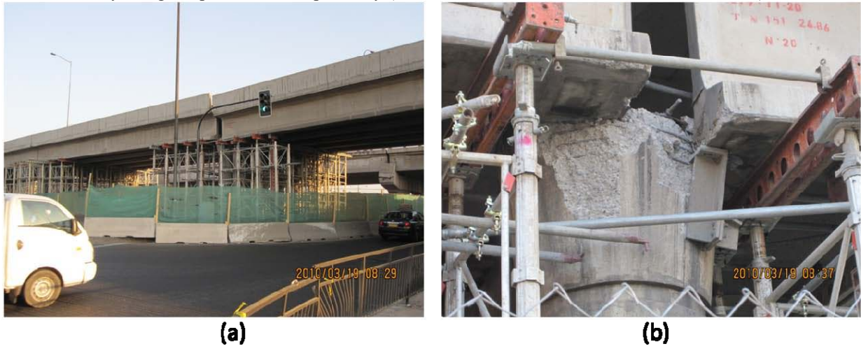
Figure 9.36 (a). Example of one of the newer under crossings that suffered damage along the Vespucio Norte Expressway. The right span became unseated due to excessive transverse movement (S33.36245, W70.688865; 829 hrs on 3/19/2010) (b) Close-up of shear key area on bent cap, with metal shear key or keeper bar hanging on right side of bent cap. Note complete unseating of I-girder on right side of bent cap (S33.366638, W70.689301; 837 hrs on 3/19/2010).
