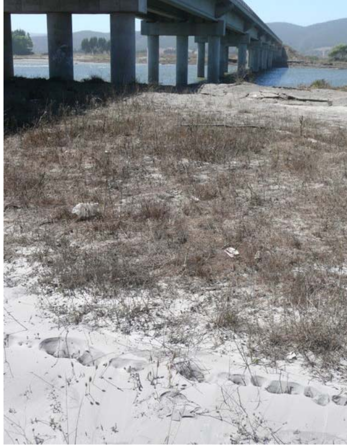
Figure 6.15. Ejecta in the foreground and lateral spreading cracks in the back ground along the south landing of the Mataquito bridge (S3505078°, W72.16240°, 11:00, 3/8/2010).
