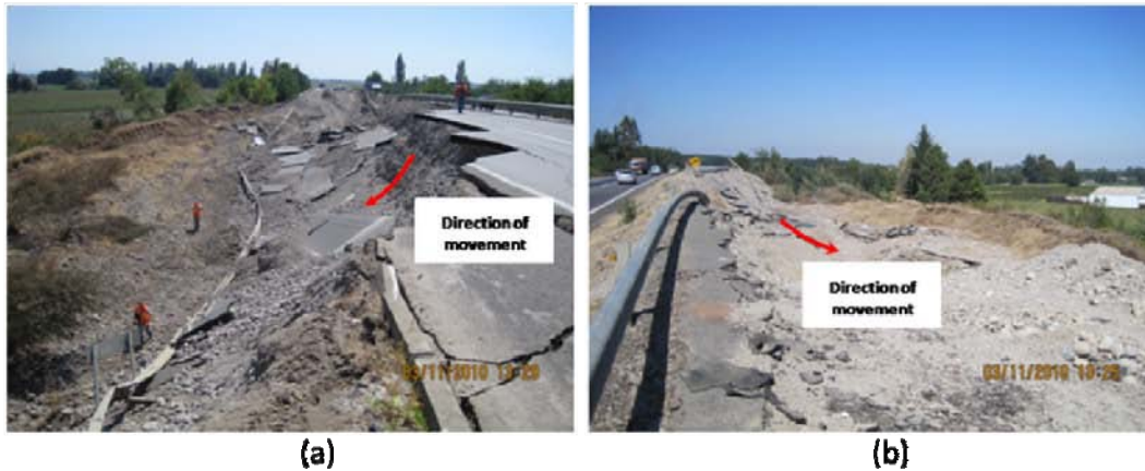
Figure 9.57. This embankment fill collapsed together with an overhead near Copihue, north of Parral, closing the South bound of Route 5 (a) View from the South, (b) View from the North (S36.087891, W71.791513, 1325 hrs on 3/11/2010)
