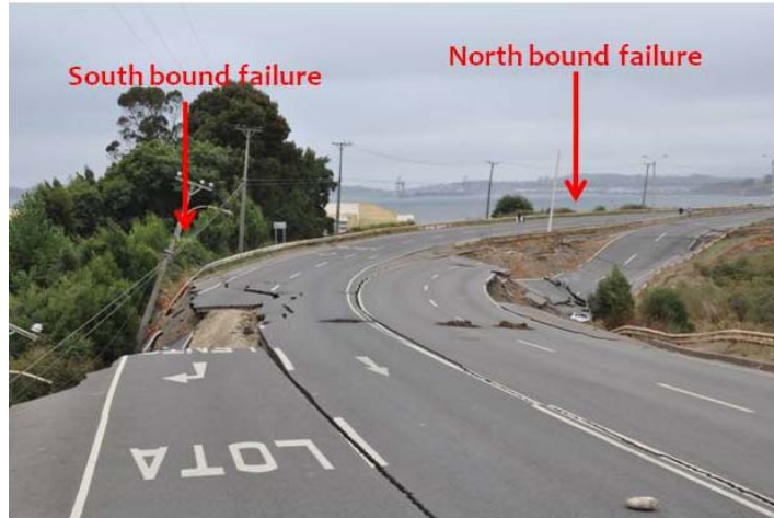
Figure 9.54. View looking north on route 160 showing south bound and north bound failure areas (S37.0744°, W73.1480°; 1220 hrs on 3/16/2010).
