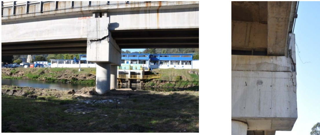
Figure 9.22. Damage to transverse shear keys at bent #3 due to movement of the La Mochita bridge (S36.847405°, W73.055084°; 1830 hrs on 3/15/2010).
