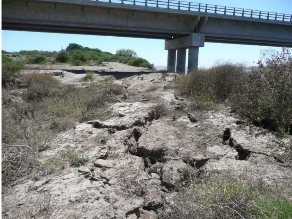
Figure 6.13. Lateral spreading at the south landing of the Mataquito bridge along the coastal highway (S3505078°, W72.16240°, 11:00, 3/8/2010).
