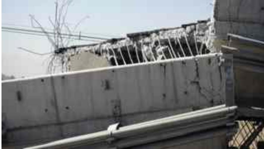
Figure 5.8. Paso Miraflores (S33.3945° W70.7700°). Deck collapse detail (Source: Dr. Roberto Leon, personal communication).
