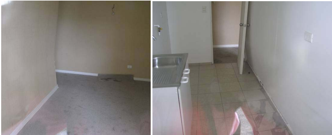
Figure 7.21. Evidence of interior damage to Riesco Building due to differential foundation movement (S36.79085°, W73.08128°; 1320 hrs on 03/17/10).
