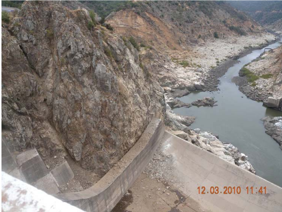
Figure 10.2. Rock fall from the downstream left abutment of Rapel Dam (34.04167°S, 71.59263°W).
