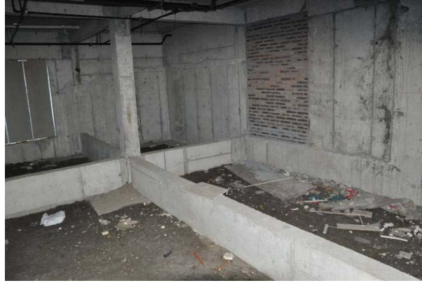
Figure 7.6. General configuration of the foundation, perimeter structural shear walls and interior gravity columns (view at ground floor of wing 2I looking east) (S37.47366°, W73.34761°; 1625 hrs on 3/16/2010)
