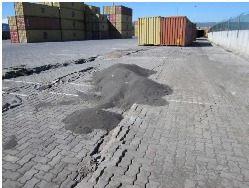
Figure 1 Sand Ejecta, Lateral Spreading, Port Coronel, April 14, 2010 (37.028874°S, 73.149768°W).
