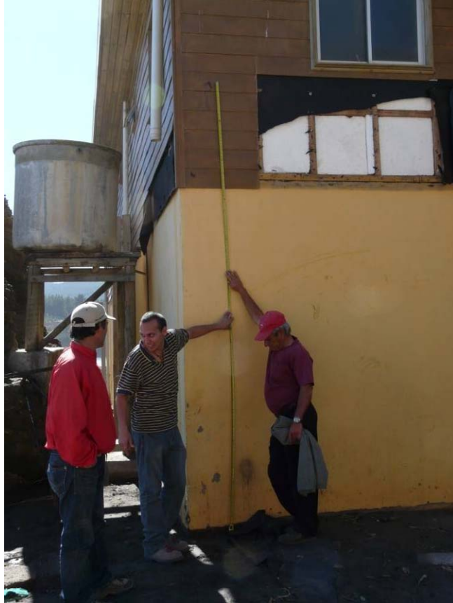
Figure 13.27. Damaged siding on this building suggests tsunami flow depths reached at least 3.5 m at the west end of Bucalemu (S34.640097° W72.044194°, 1130 hrs on 03/15/2010).
