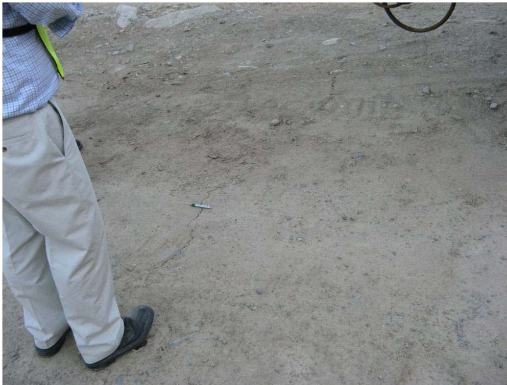
Figure 11.19. March 10, 2010 Millimeter Width Transverse Crack Near the Left Abutment of Caren Tailings Dam (S34.096050°, W71.180748°)
