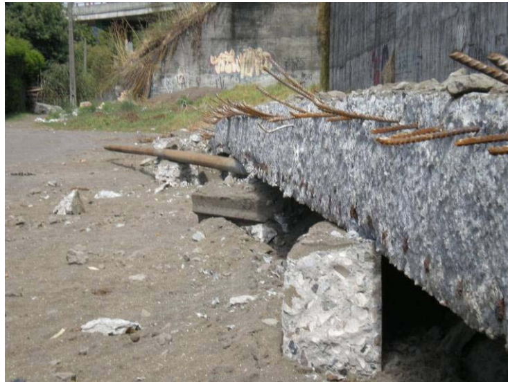
Figure 12.8. Toppled portion of 16-inch thick wall showing bent compression bars and snapped tension bars.
