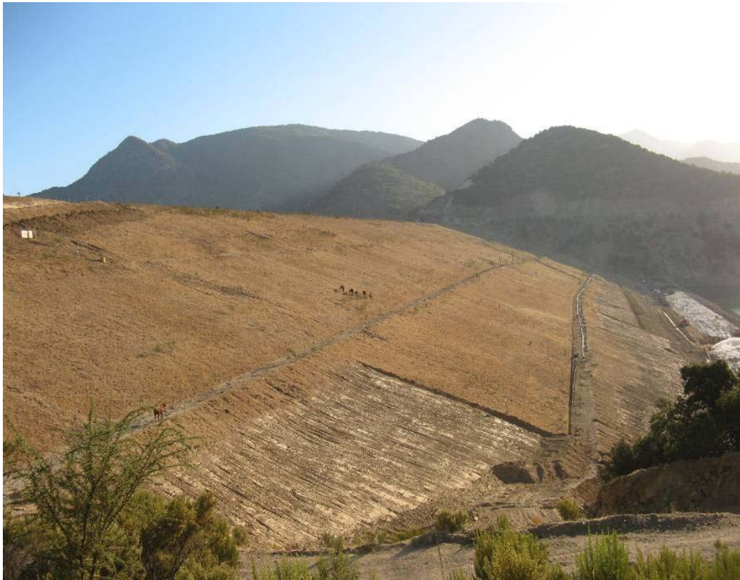
Figure 11.20. March 10, 2010 View of the Downstream Face of the Caren Tailings Dam Showing Progress of Dam Raise Construction (S34.092422°, W71.173250°)
