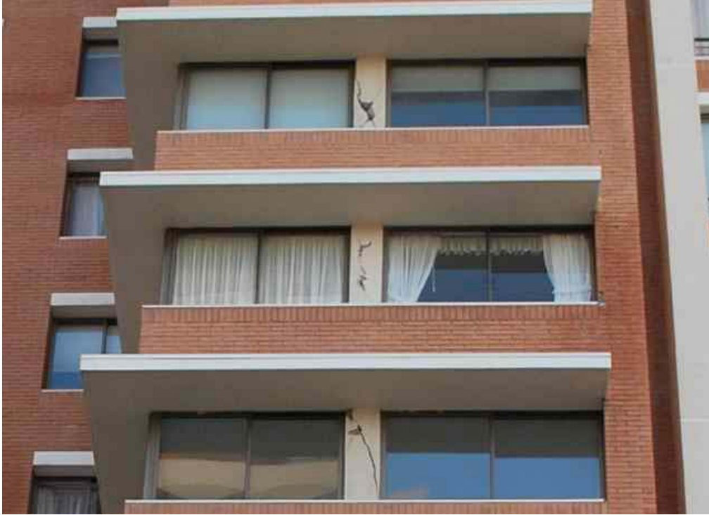
Figure 5.25. Site DA020 (S 33.018678° W 71.556288°, 1953 hrs on 03/14/2010). Diagonal cracks of columns in all the floors of 19-story building.
