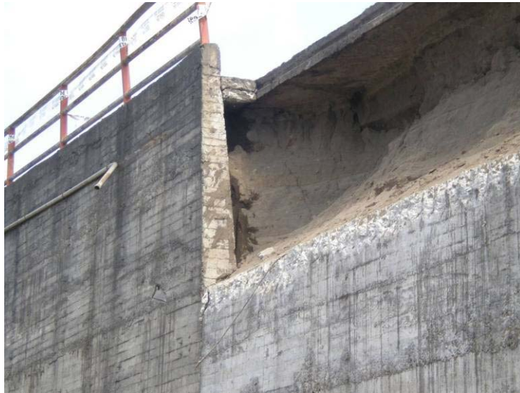
Figure 12.9. Granular fill soils and water seepage evident behind failed portion of wall.
