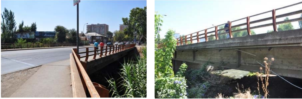
Figure 9.30. (a) Typical short span bridge construction on the branch of the Rio Claro, city of Talca (S35.428011° W71.670269°; 1302 hrs on 3/18/2010). (b) Bridges were observed to remain undamaged (S35.428086° W71.669894°; 1303 hrs on 3/18/2010).
