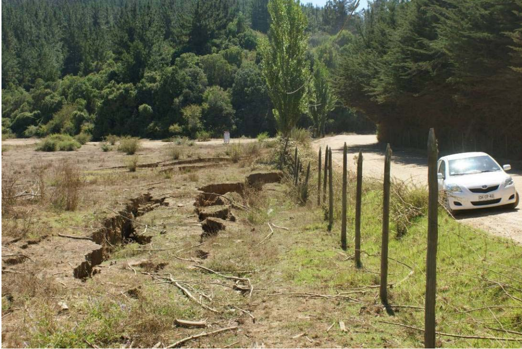
Figure 14.12. Lago Vichuquen,. Lateral spreading on the inland side of the lakefront road. (S34.39097°, W72.077815°; 12:46 hours on 3/15/2010)
