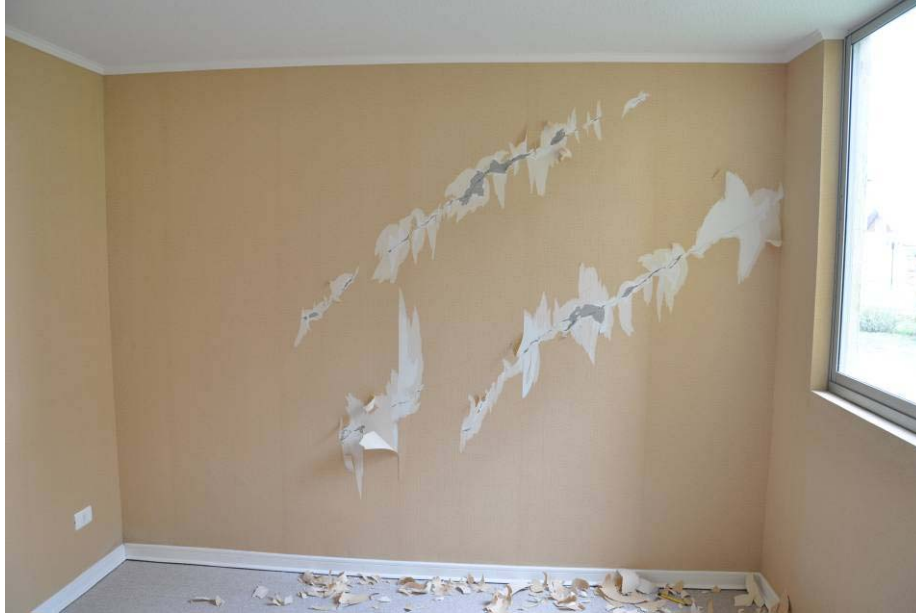
Figure 7.25 Damage to ground floor shear walls of the Montt building (S36.790737°, W73.080901°; 1545 hrs on 3/17/2010)
