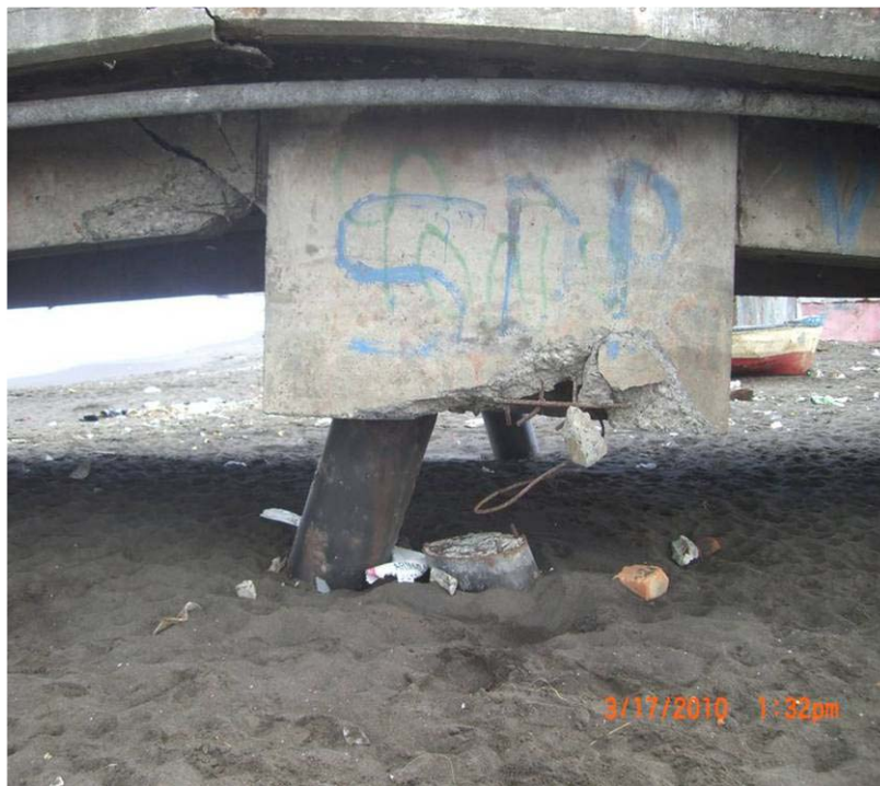
Figure 8.13. Photograph of pile cap with battered piles supporting pier at small fishermen's Port of Coronel showing pull out of trailing row piles (S37.024319°, W73.156210°; 1322 hrs, 03/17/2010).
