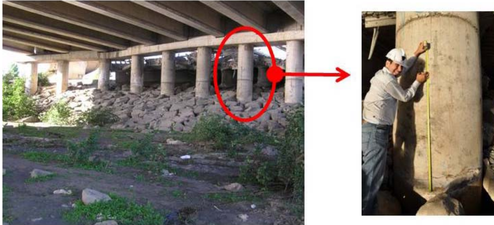
Figure 9.6. Substructure of the north approach at the damaged Llacolén bridge in Concepción showing the unseated deck in the foreground. Flexural cracking of the column supports was observed at ground level and extending to the construction joint (2-2.5m above ground)
