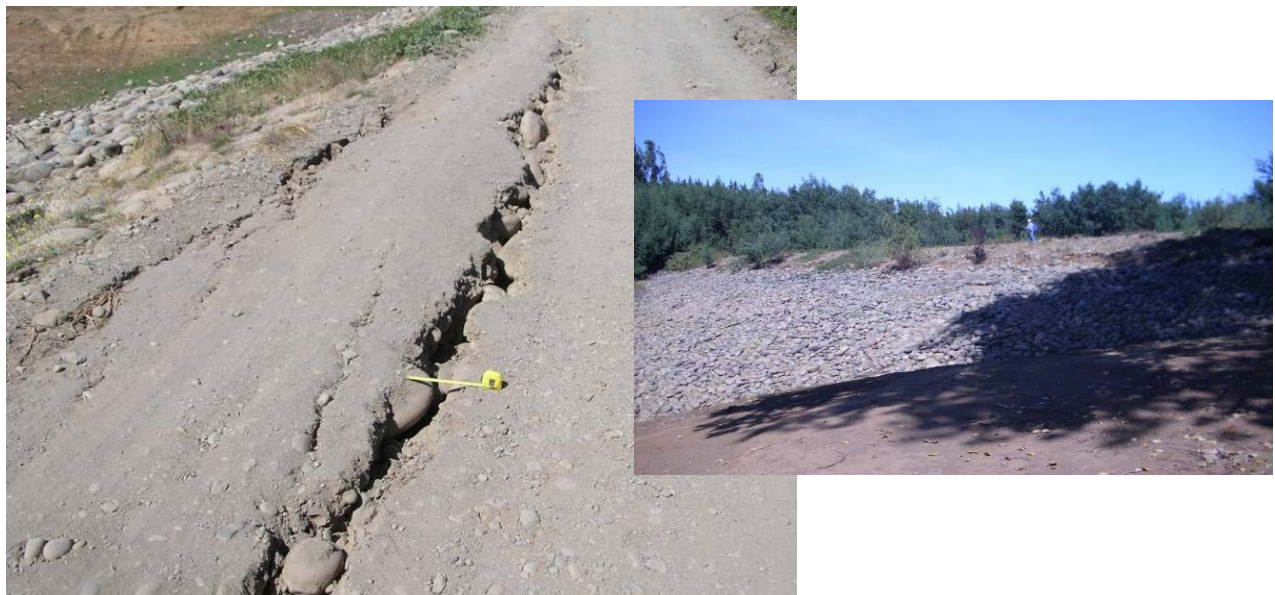
Figure 11.5. March 10, 2010. Cracking of Crest of Small Dam South of Main Coihueuco Dam (S36.645411°, W71.800212°).
