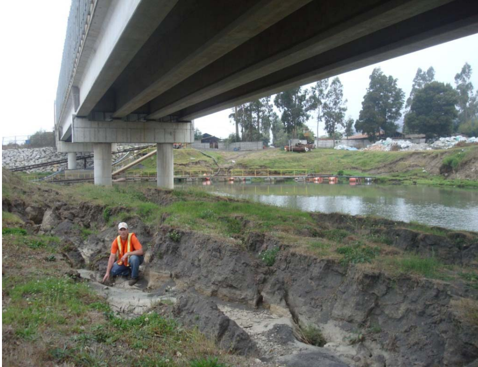
Figure 15.27. Liquefaction-induced lateral spread at Concepcion bridge parallel to the Bio Bio River. (36.84722°S, 73.05530°W; 27 March 2010; 09:25)
