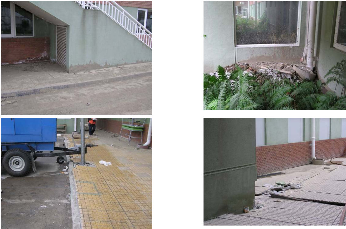
Figure 7.7. Sediment ejecta observed around hospital wings; (a) ejecta observed along exterior staircase of Wing 1D (S37.47358°, W73.34890°), (b) ejecta observed along exterior of Wing 1C (S37.47342°, W73.34829°), (c) ejecta observed along south side of Wing 1D(S37.47375°, W73.34851°), and (d) ejecta observed along east side of Wing 2G (S37.47343°, W73.34788°).
