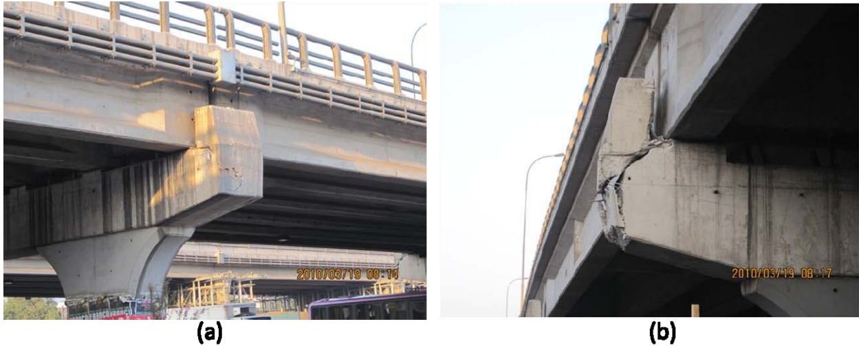
Figure 9.35. (a) Damaged shear key is an example of typical performance on bridges along this section of Vespucio Norte Expressway in Quilicura (S33.365585, W70.688657; 814 hrs on 3/19/2010), (b) Close up of damaged shear key along Vespucio Norte Expressway (S33.365893, W70.688584; 817 hrs on 3/19/2010).
