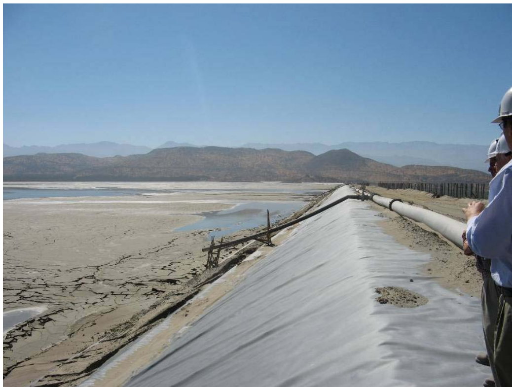
Figure 11.10. March 9, 2010 View along the Upstream Face of the Ovejeria Tailings Dam. There is no damage to the liner and no signs of slumping of the sand beneath the liner (S33.052911°, W70.807067°)
