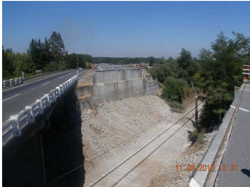
Figure 12.2. Reinforced Earth bridge abutments at a collapsed rail crossing on Route 5 north of Parral (36.0803°S, 71.788°W)
