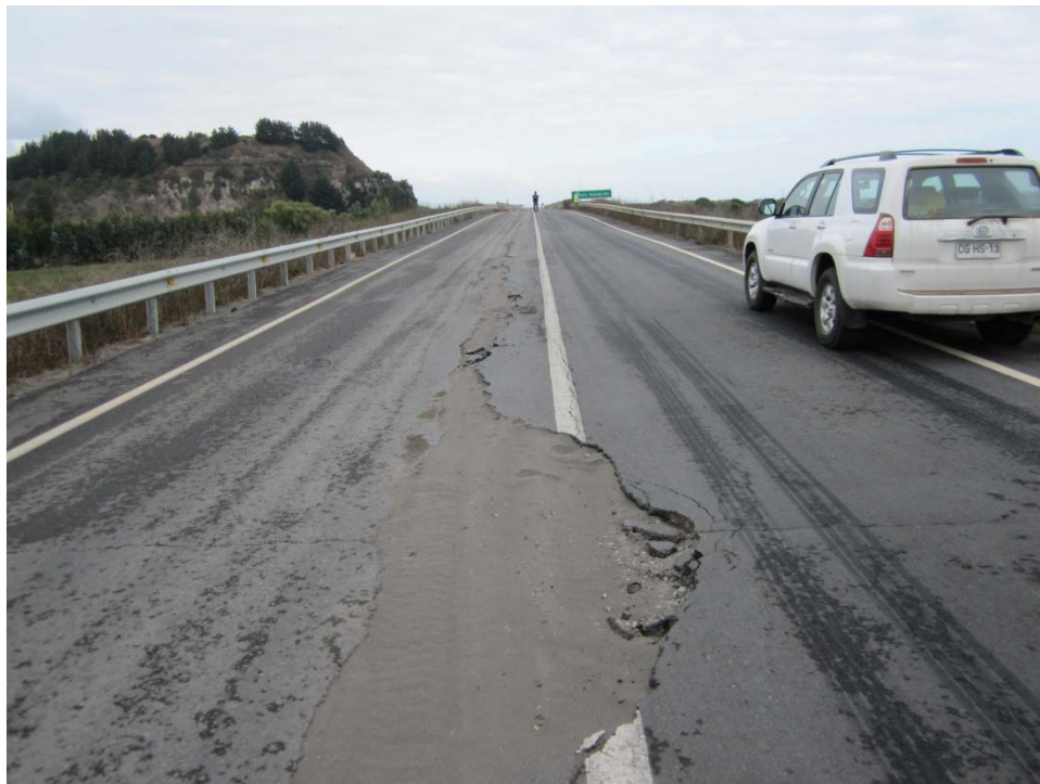
Figure 15.67 Cracking and transverse movement (60 cm on each side) of embankment due to liquefaction of underlying soil, north abutment of the bridge, Puente Mataquito, 35.050712°S, 72.162258°W, April 16, 2010.
