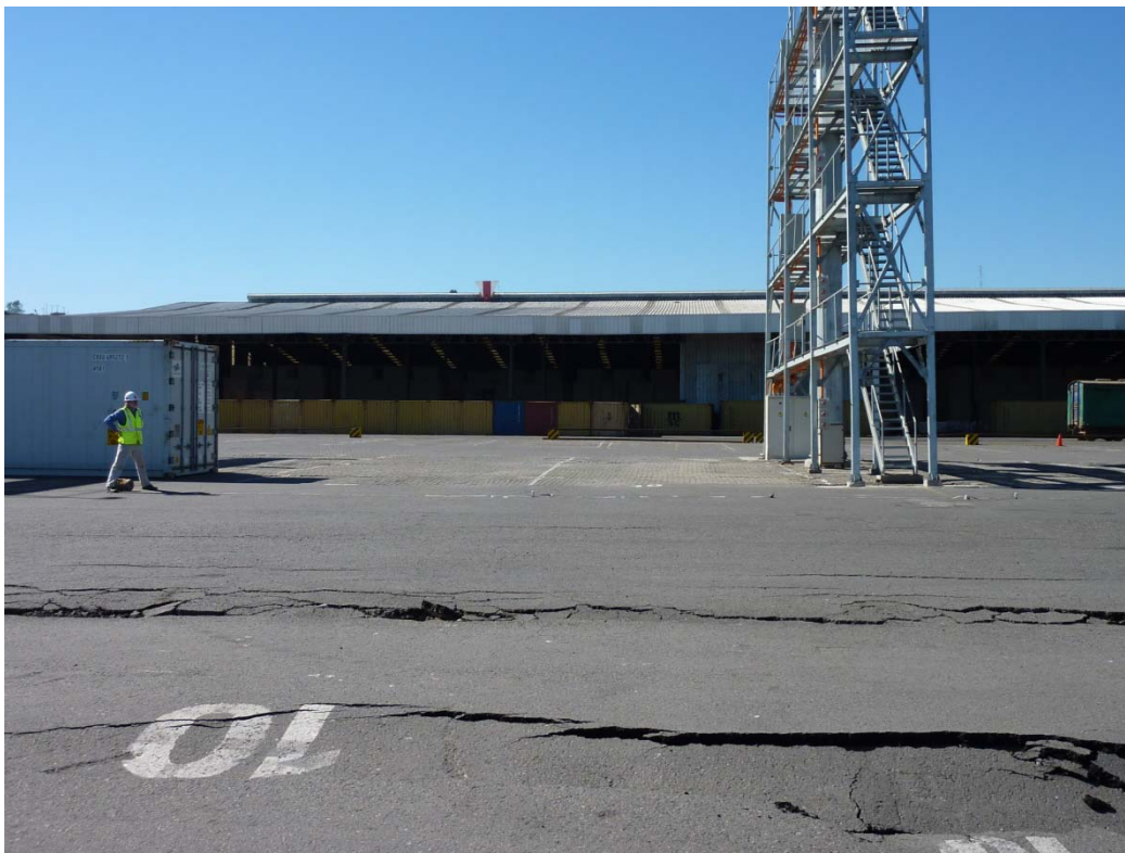
Figure 15.75 SASW line 2, and lateral spreading looking north, Port Coronel, April 14, 2010 (37.028874°S, 73.149768°W).
