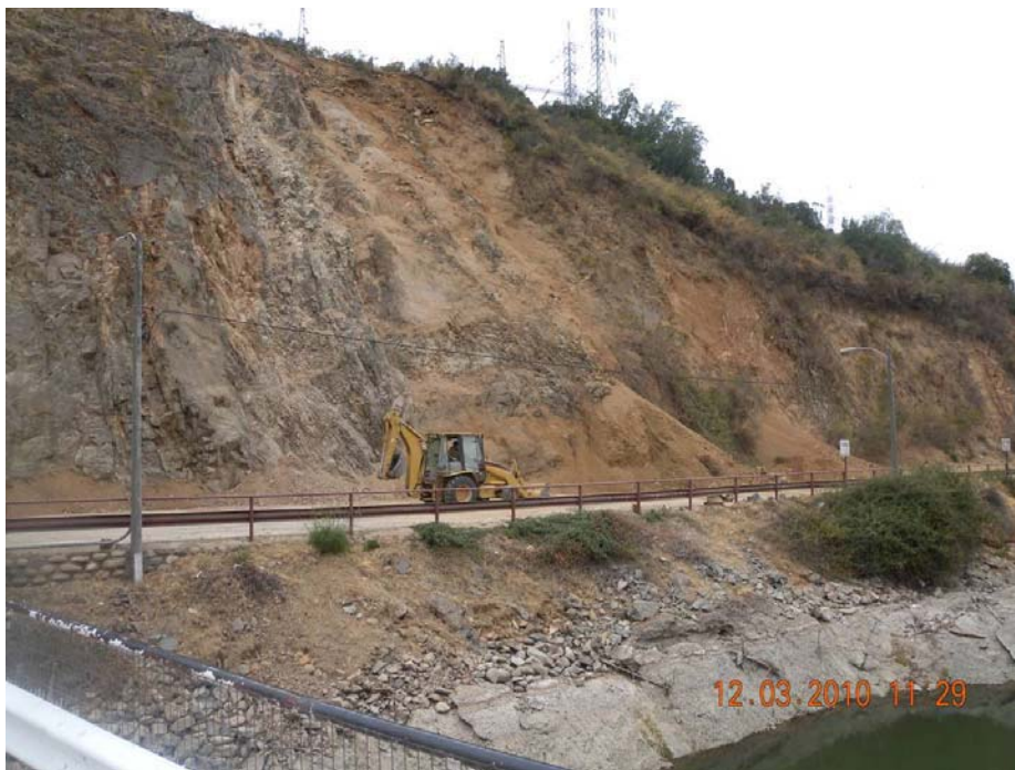
Figure 10.3. Shallow raveling failure of a road cut in weathered and heavily jointed granitic rock at Rapel Dam (34.0407421°S, 71.587153°W).
