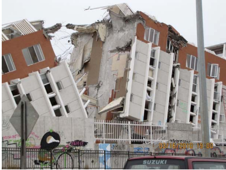
Figure 5.34. Collapsed structure (S 36.828067° W73.061639°, 1900 hrs on 03/16/2010) designed using Soil Type II conditions.
