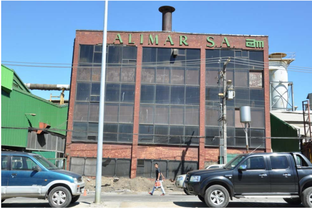
Figure 8.24. Damage to fish packaging facility (S36.7260°, W73.1288°; 1345 hrs, 03/15/2010).
