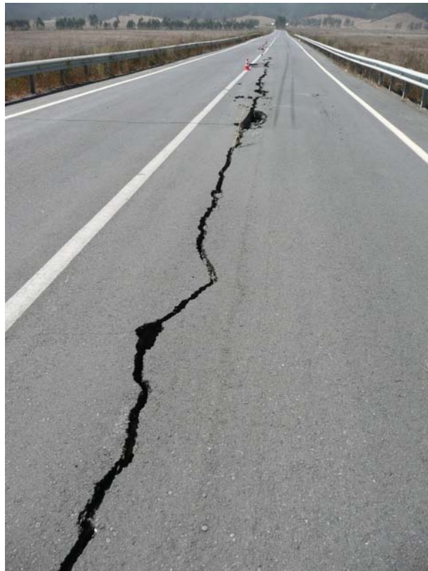
Figure 6.12. Impact of liquefaction and lateral spreading on the north approach fill of Mataquito Bridge (S3505078 °, W72.16240°, 11:00, 3/8./2010).
