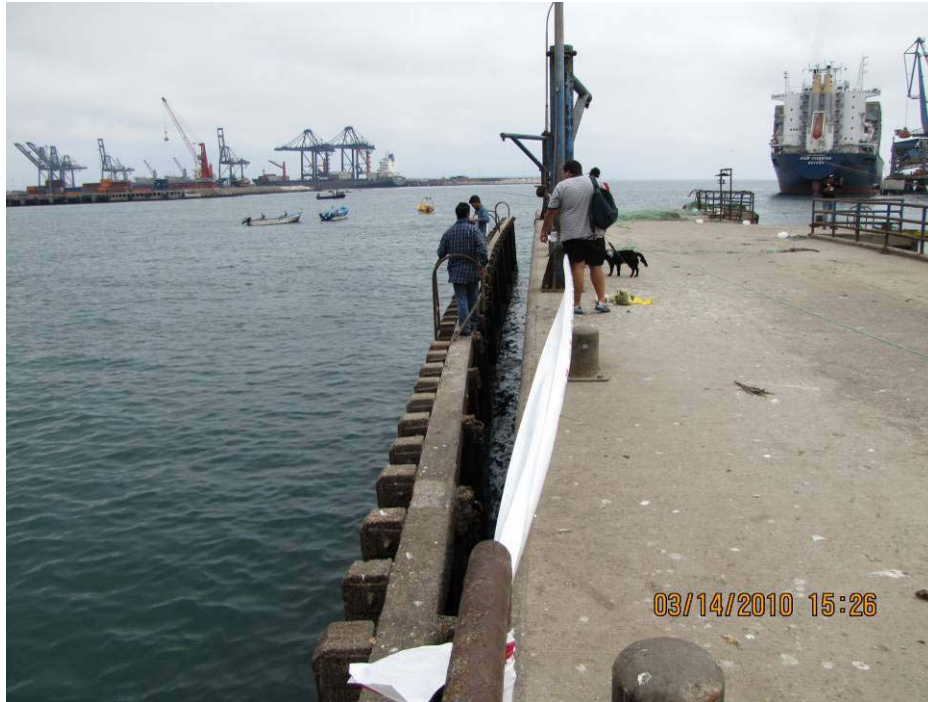
Figure 8.35. Separation from lateral pile screen of wharf structure in San Antonio Port (S33.5817°, W71.6154°; 1526 hrs, 03/14/2010).
