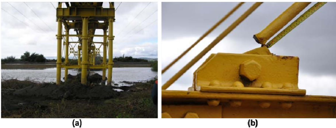
Figure 9.26. Bio Bio Railroad crossing (a) Pillars move and rotated during earthquake (b) Detail of broken crossbar, (S36.836075° W73.086969°; 1717 hrs on 3/17/2010)
