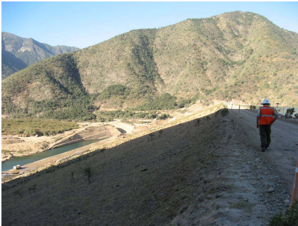
Figure 11.21. March 10, 2010 Crest and Downstream Face of Caren Dam from Left Abutment (S34.095570°, W71.179076°)
