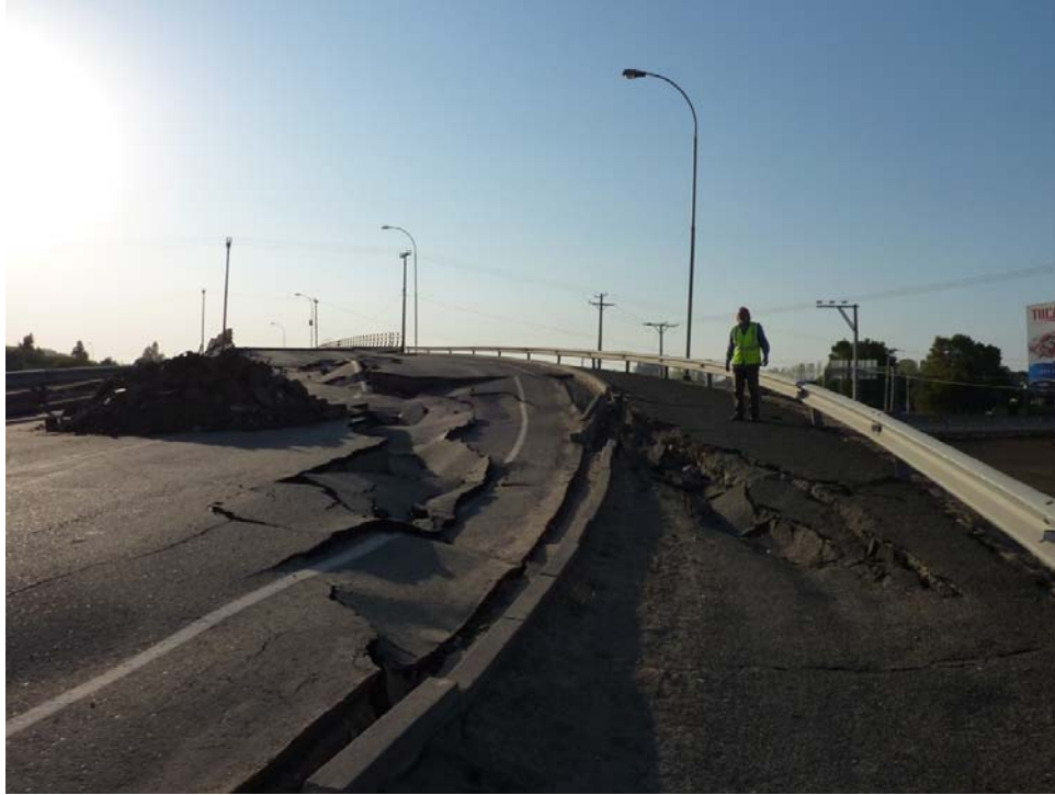
Figure 15.83 Damage to over padded embankment, Ruta 5 Sur overpass embankment, to Retiro at Tucapel Mill, April 15, 2010 (36.051209°S, 71.768005°W).
