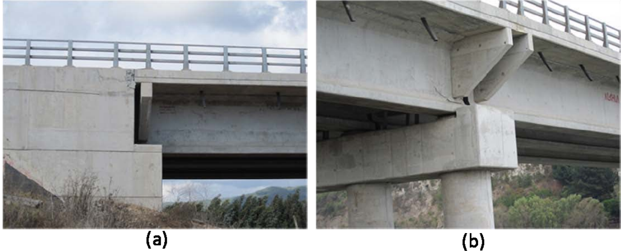
Figure 9.43 (a) North abutment shoved into bridge deck due to lateral spreading, Puente Mataquito, S35.050712°, W72.162258°, April 16, 2010, (b) Shearing of bridge girder, North abutment of bridge, Puente Mataquito, S35.050712°, W72.162258°, April 16, 2010.
