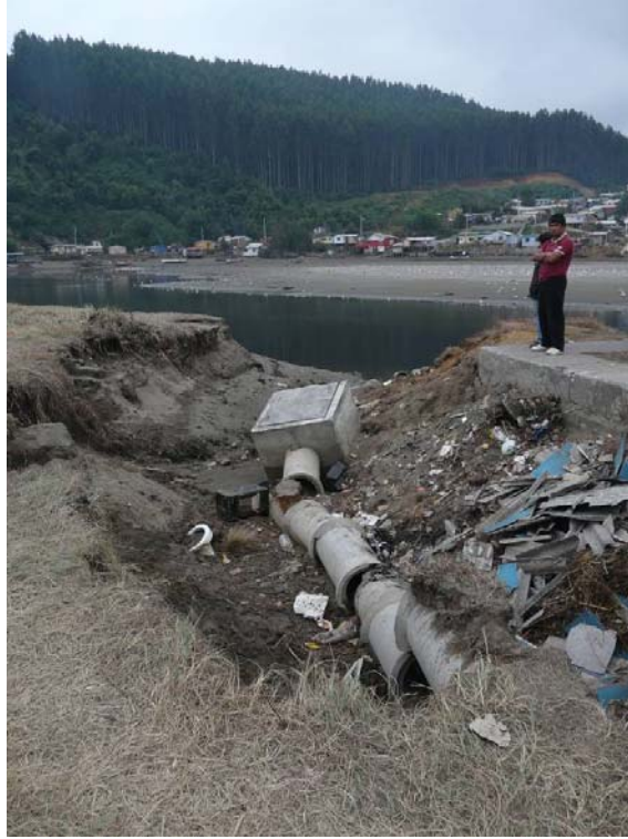
Figure 13.1. Tsunami scoured out the foundation of this storm sewer outfall at Laraquete (S37.165352° W73.188051, 1907 hrs on 03/16/2010).
