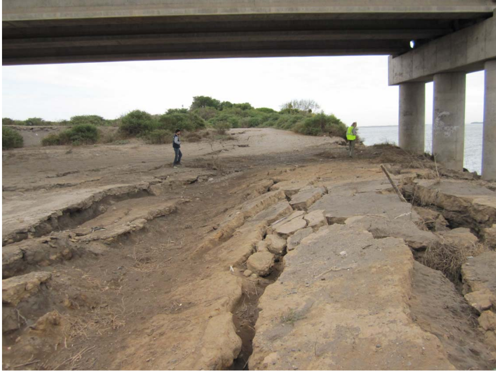
Figure 15.64 Lateral spreading on the south end of the bridge, Puente Mataquito, 35.050712°S,72.162258°W, April 16, 2010.
