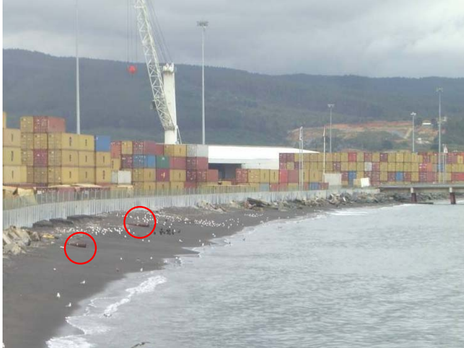
Figure 8.6. Pipelines running transverse to sheet-pile wall which were subjected to longitudinal strain due to lateral spreading (S37.028680°, W73.150054°; 1520 hrs, 03/17/2010).
