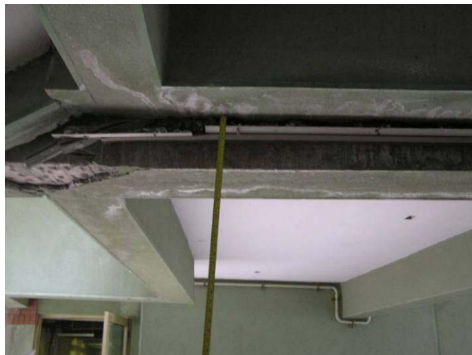
Figure 7.10. Relative movement between Wing 1B (in the background) and Wing 2G (in the foreground) (S37.47335°, W73.34786°; 03/16/10).
