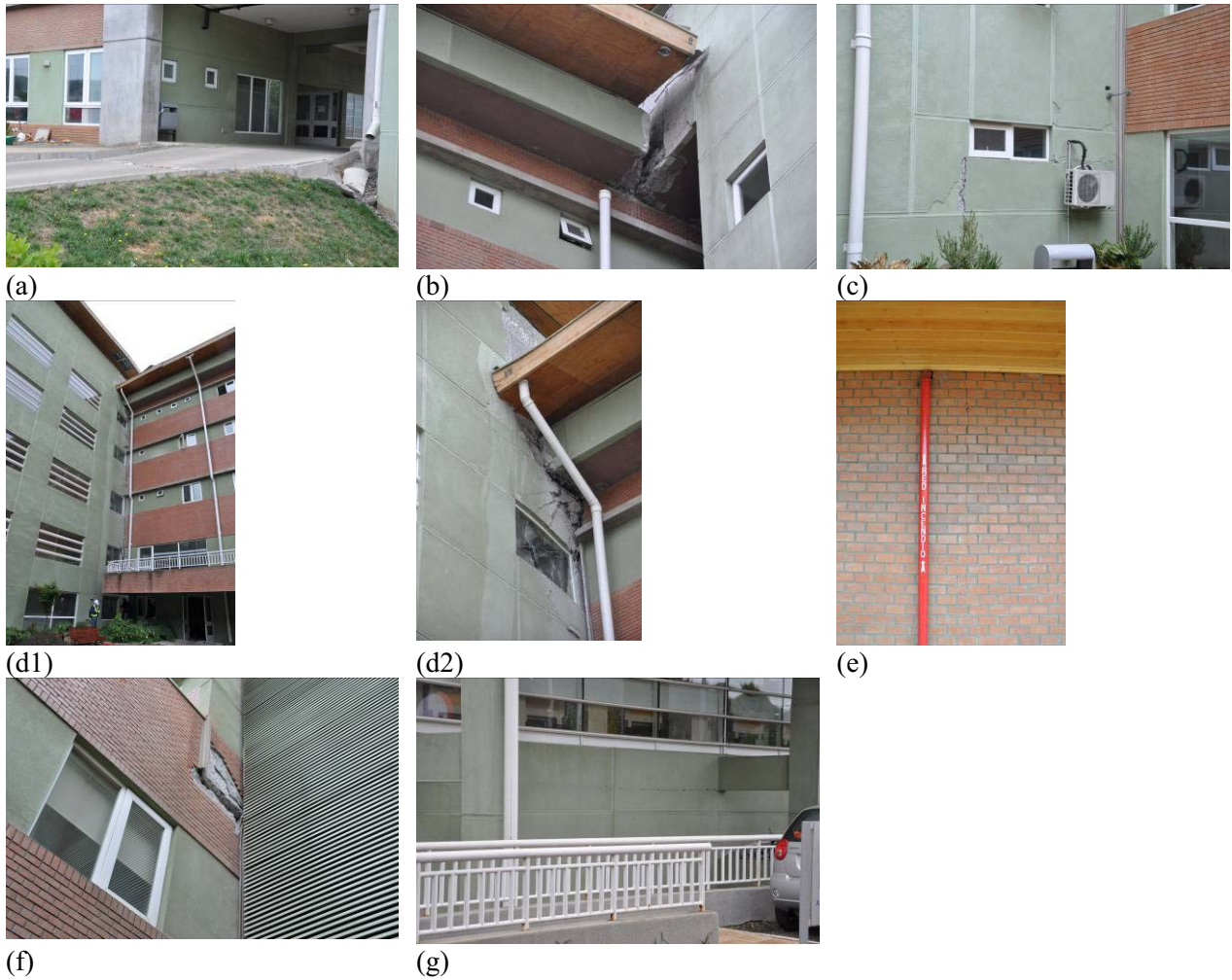
Figure 7.12 Most pronounced structural damage observations. (a) approach ramp to entrance bay at wing 1A (S37.473084°,W73.348712°), (b) pounding damage and resulting permanent gap developed between wings 1A-1C due to the easterly rocking of wing 1C (note the gap was measured by hospital staff as 37 cm after the main event on February 27, 2010) (S37.473376°, W73.348452°), (c) damage to shear wall of wing 1C due to contact with wing 1D (S37.473537°, W73.348488°), (d1) elevation view of the interface between wing 1B-1C and (d2) local view at the roof line of wing 1B observing the pounding between these two wings (S37.473406°,W73.348304°), (e) vertical cracks in masonry in-fill of wing 2H (S37.473713°, W73.347839°), (f) fallen masonry façade and spalling of structural wall of wing 1F due to impact with wing 1B (S37.473494°, W73.347948°), and (g) cracking damage at in-fill and structural shear wall interface at front of wing 2I-2J (S37.473528°, W73.347363°). Images taken at 1430, 1715, 1415, 1725, 1725, 1350, 1625, and 1645 hrs, respectively, on 3/16/2010.
