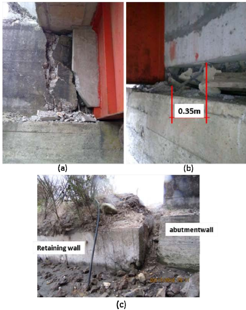
Figure 9.51. Damage to bridge abutment due to lateral spreading of soil around bridge abutment. (a) abutment wall movement relative to beams, (b) deformation of vertical restraining bar due to abutment movement relative to beams, (c) movement of retaining wall relative to abutment. (S37.254345°, W73.437021°; 1911 hrs on 3/17/2010)
