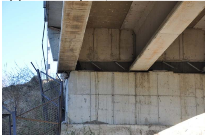
Figure 9.20. Transverse shift of deck relative to south abutment at the La Mochita bridge (S36.847547°, W73.054876°; 1834 hrs on 3/15/2010).
