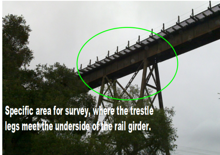
Figure 6-2 The connection point of the trestle and the girder is the focal point of study with the remote vehicle, as viewed to the south southwest, from road level.
