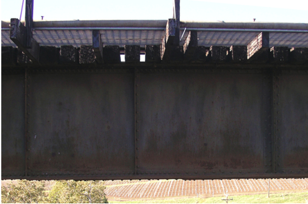
Figure 7-6 A close up cropped and rotated version of Figure 7-5, note the orange fiber optic cable conduit on the upper left center.
