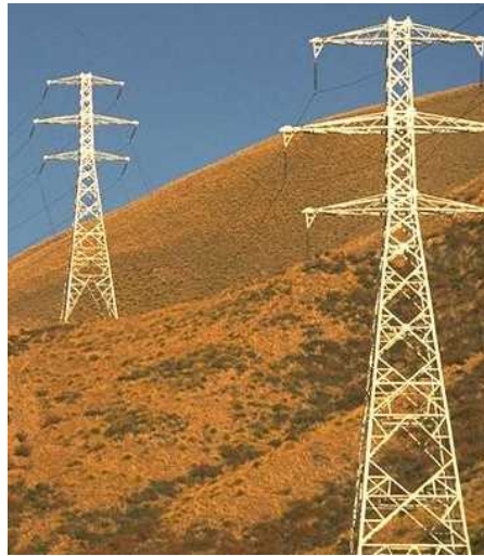
Figure 5-2 Three phase alternating current transmission towers.
