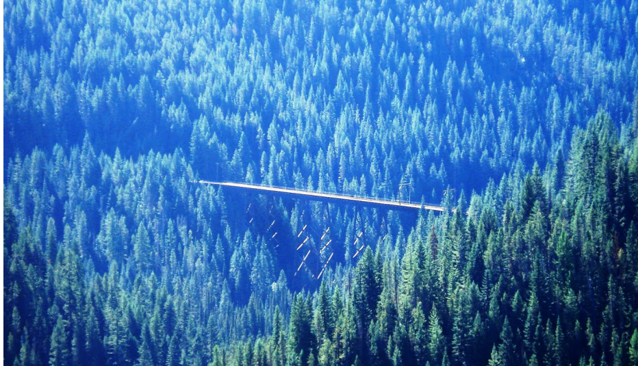
Figure 5-1 Kelly Creek Trestle, Montana, 260 meters long, 70 meters high. An example of a bridge structure that could benefit from quick, inexpensive, survey techniques.
