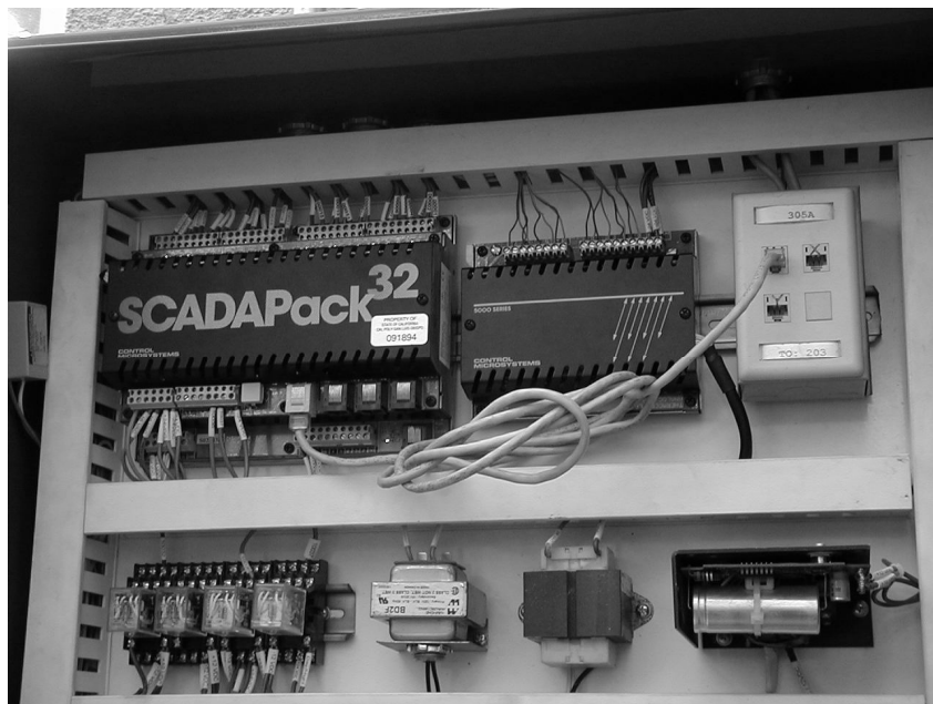
Fig. 2. SCADAPack 32 and auxiliary components.
