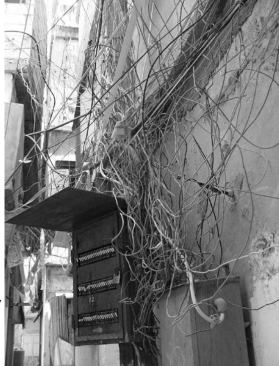
Figure 3.3: Electrical wires tapping into a power main- Burj El Barajneh
