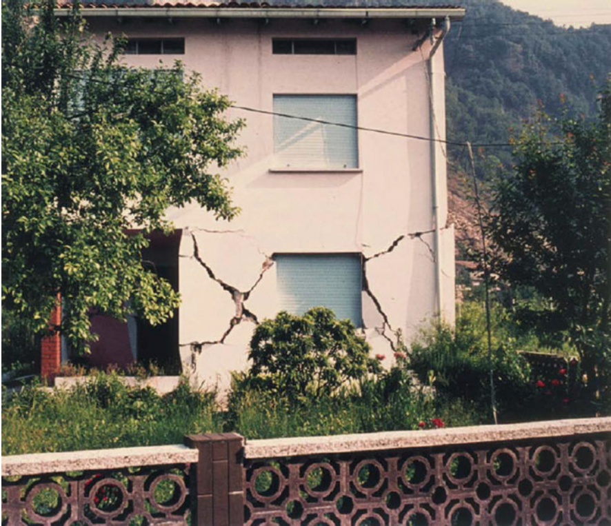
Fig. 16.7 Unreinforced masonry with RC floors, grade of damage 4 (Grünthal 1998, EMS-98 scale)
