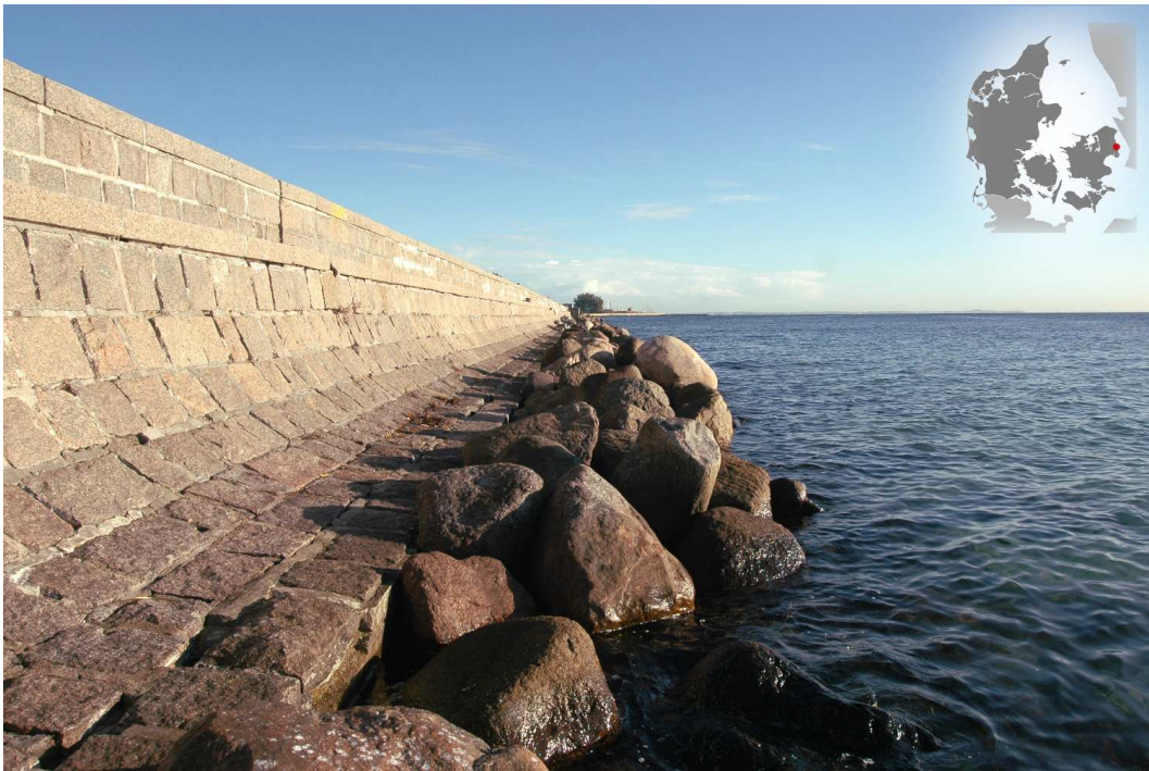
Figure 1.6: Seawall fronted by a revetment at Charlottenlund, Denmark. Seawalls force the water depth at the structure to increase in response to erosion. Photo by author, September 2012.
