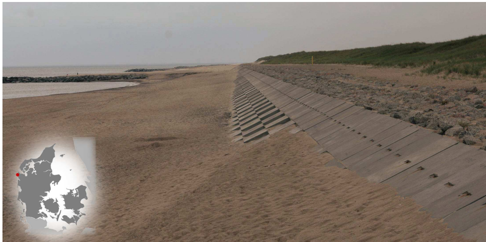
Figure 1.7: A buried revetment at the West Coast of Denmark, which is intended as armouring of the dune during storm conditions. Photo by author, June 2010.
