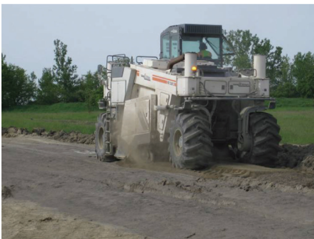
Figure 4.6 Mixing of steel slag-fly ash mixture with the in situ subgrade soil.
