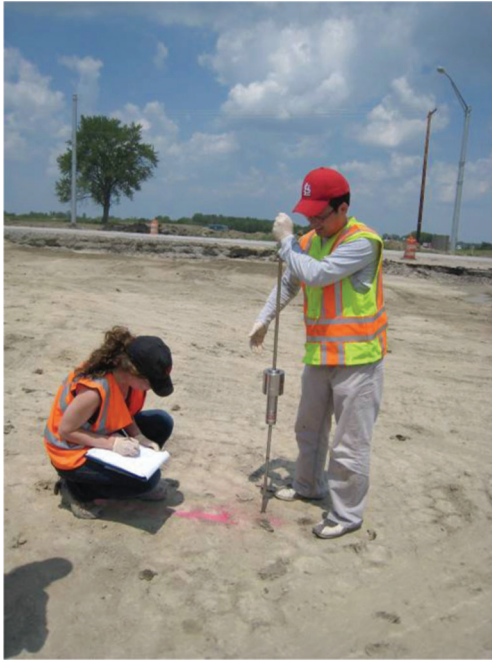
Figure 4.12 Dynamic cone penetration testing of the subgrade soils stabilized with 7% steel slag-3% Class-C fly ash mixture.
