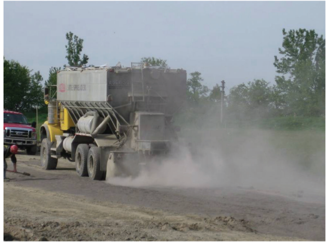
Figure 4.3 Spreading of the steel slag-Class-C fly ash mixture on the subgrade soil.
