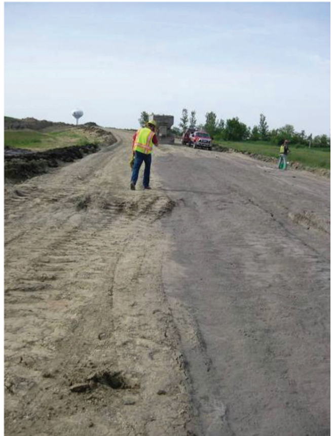
Figure 4.4 View of the ramp section after the spreading of the steel slag-Class-C fly ash mixture.
