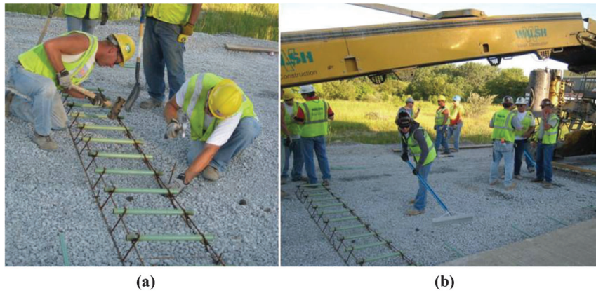
Figure 4.13 Pavement work prior to placement of concrete: (a) placement of reinforcement and (b) leveling of the base course.
