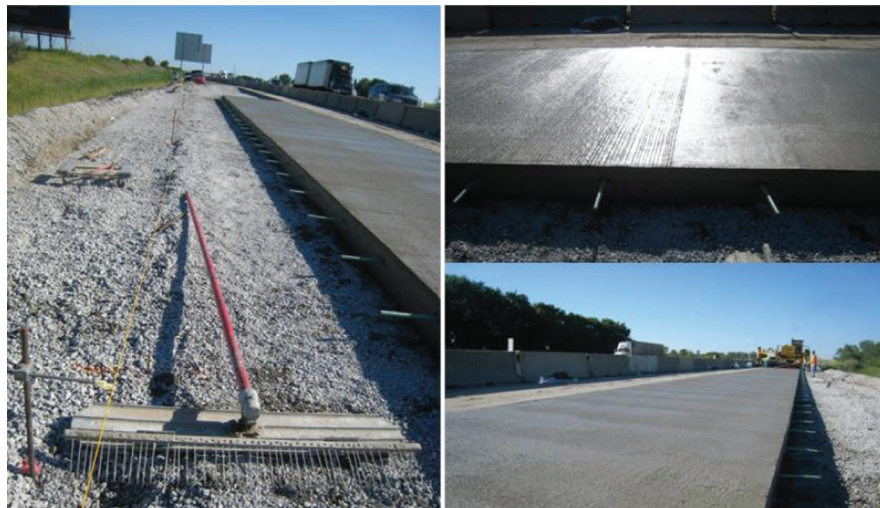
Figure 4.17 Tinned concrete surface.
