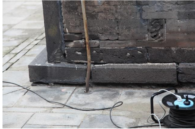
Figure 19 Settlement of the pedestal of the temple gate
