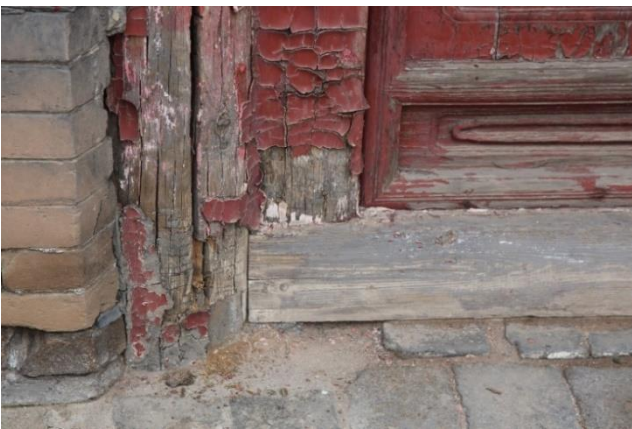
Figure 15 pillar cracks of the temple gate
