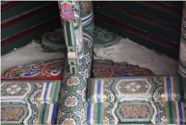
Figure 14 Wooden structure cracks of the temple gate
