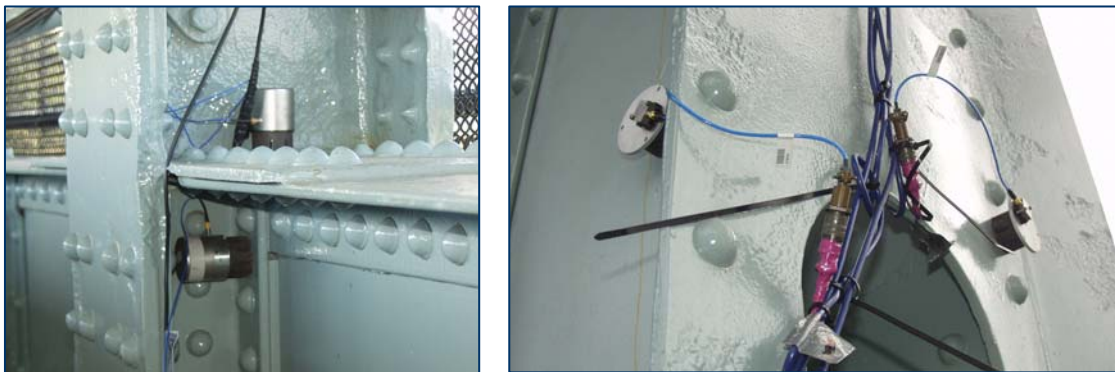
Figure 5-11 Vertical and transverse on the lower deck level of the arch span (left); Transverse and longitudinal sensors on the tower (Right)
