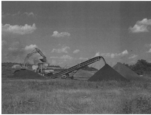
Fig. 2. Overview of pugmilling operation and CG–DM blend stockpile generation using a radial stacker
