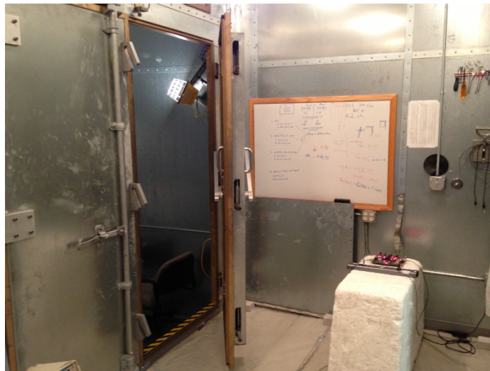
Figure 4.14: Position of the shielded door between the main chamber and the ante chamber for High Coupling configuration.
