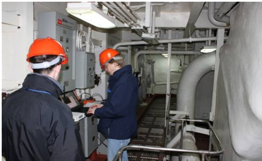
Figure 1.1: Engine Room on the Thomas S. Gates (CG 51).
