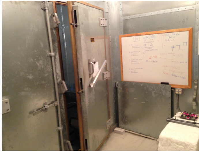
Figure 4.13: Position of the shielded door between the main chamber and the ante chamber for Medium Coupling configuration.
