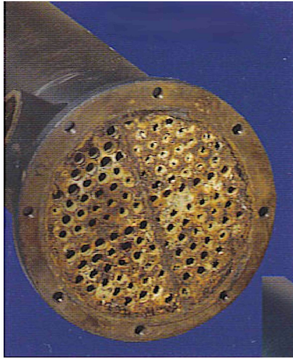
Figure 7. Typical severe condenser tube fouling.
