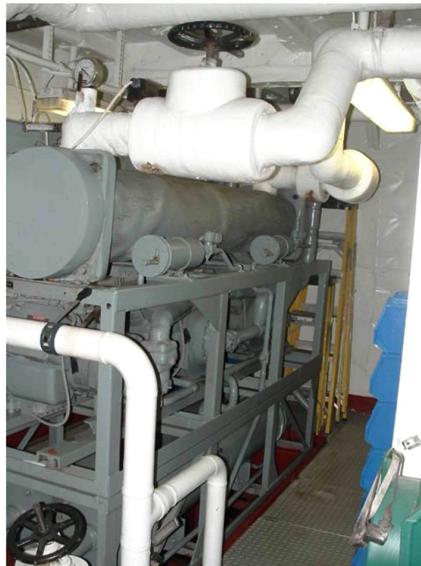
Figure 6. STBD A/C Chiller Plant
