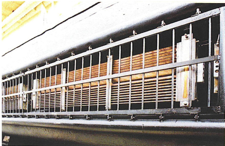
Figure 8. Typical Grid Cooler installation in side of a river boat.
