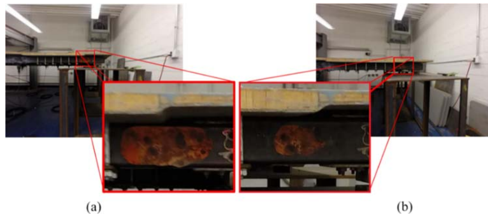
Figure 49. Corrosion setup on steel grid. (a) Image of the larger corrosion. (b) Image of the smaller corrosion [251].
