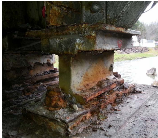
Figure 6-8: Deterioration of Exterior Expansion Bearings at Pier 1
