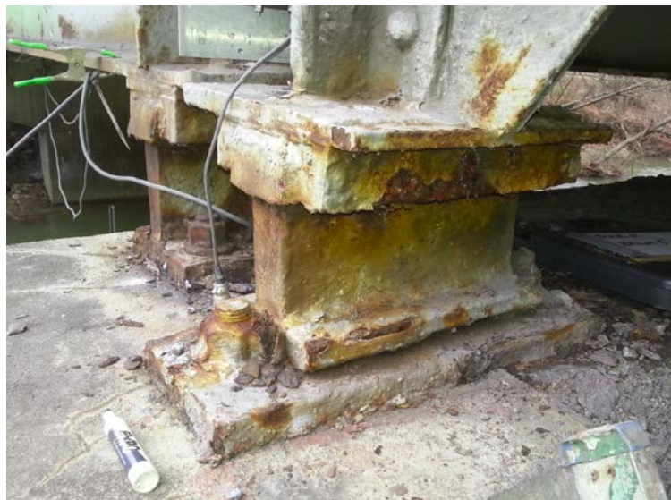
Figure 6-9: Center Span (Far) and Side Span (Near) Exterior Expansion Bearings at Pier 2
