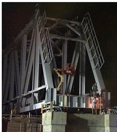
Figure 4 - Nighttime installation of a railroad bridge over I-76, just west of Philadelphia, PA.
