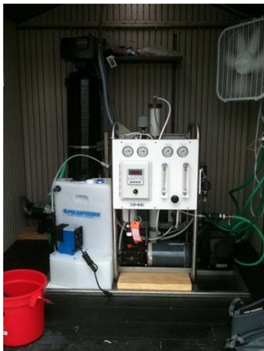
Figure 5 Mobile RO skid deployed at the Tampa Bay Seawater Desalination Plant (TBSDP; source: the author).
