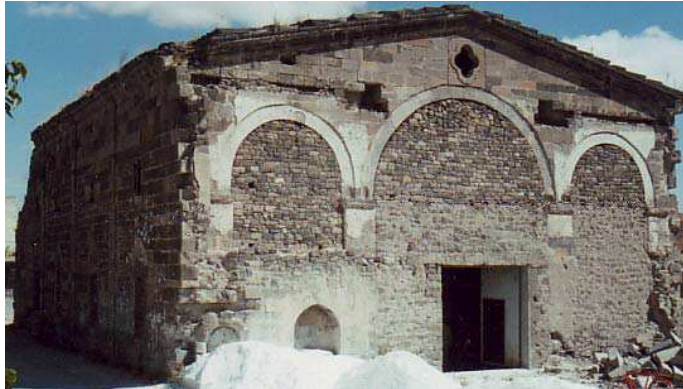
Fig.16 Tomarza Surp Boghos Bedros Church current condition. 237
