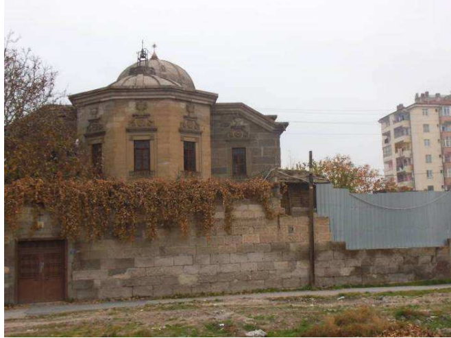
Fig. 7 The entrance façade presents partially collapsed walls. 193
