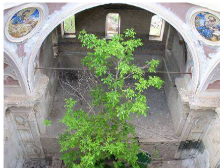
Fig.41 The absence of the dome and growing vegetation inside Surp Stepanos church of Efkere 396
