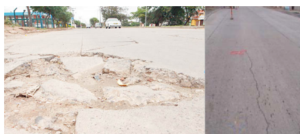
Fig. 1. A pothole and a longitudinal fissure, common in roads.
