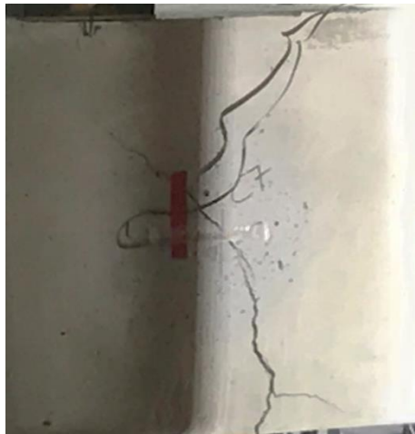
Point D. 730kN continued propagation of diagonal crack
