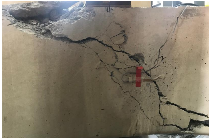
Point E. 730kN, catastrophic failure, and compression failure
