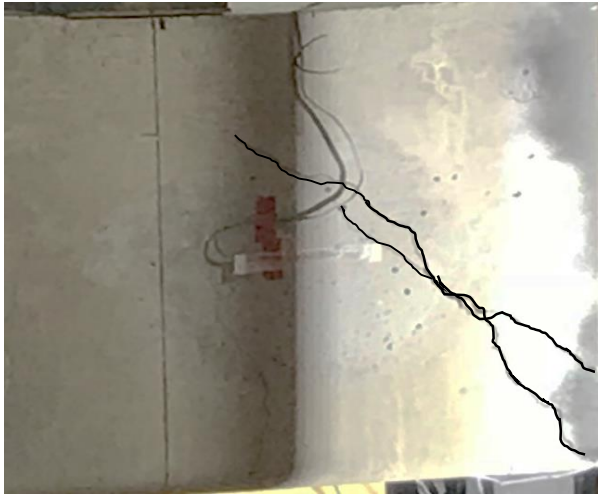
Point D. 730kN continued propagation of diagonal cracks.
