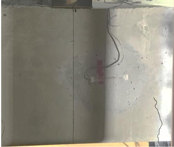
Point B. Load 400kN First Flexural Crack
