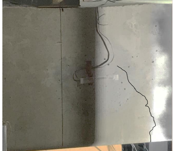
Point C. 530kN Flexural crack turns into flexure shear crack and propagates diagonally
