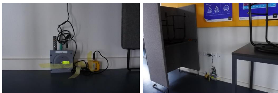
Figure 3.18: CO 2 sensor and data logger location in room 1.2.06
