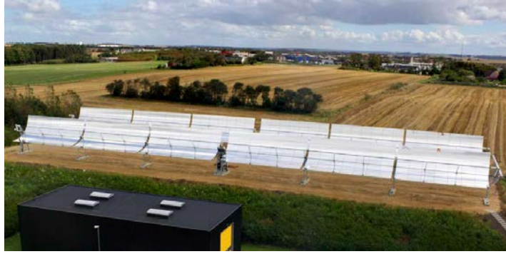
Fig. 7 The pilot parabolic trough collector loop in Thisted, Denmark (Source: Aalborg CSP A/S).
