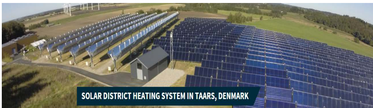
Fig. 11 The hybrid solar collector field of the Taars plant (Source: Aalborg CSP A/S).
