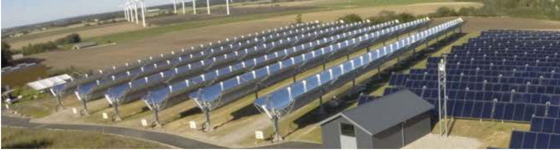
FIGURE 2. Schematic view of the plant; (b) View of the Taars plant (Denmark)
