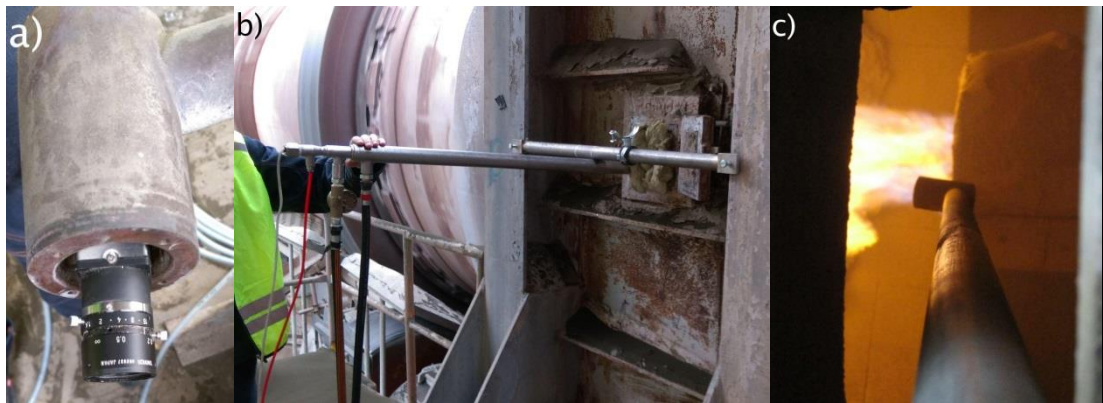
Figure 5-2: a) The camera inserted in the probe. b) Camera probe inserted through side of kiln hood. c) Camera probe inserted next to kiln burner.
