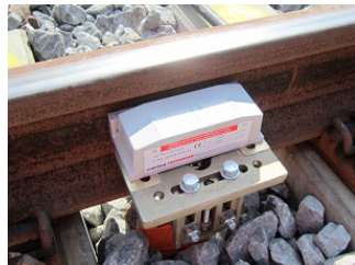
(d) Wheel detector mounted on proximity of the rail web
