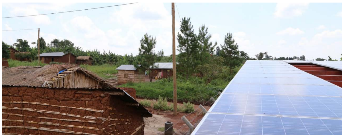
Figure 2. The 13.5 kWp installed solar mini-grid project in Kyamugarura, west of Uganda in Kyenjojo District, providing electricity to sixty local connections. The solar panels are mounted on top of two containers, which serve as an office for the cooperative.
