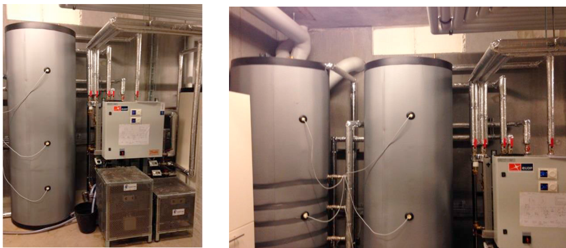
Fig. 3. (a) HBS installed in technical room; (b) Part of HBS unit with both tanks
