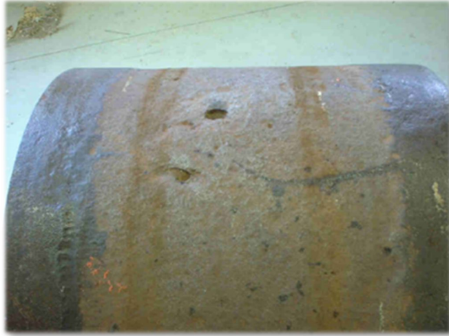
Figure 6.1: Photograph of deep, highly localised pits on the surface of a pipe located underneath a support (Burch, 2016).
