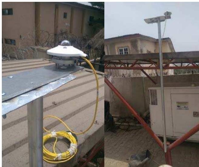
Figure 3.5: Installed Kipp and Zonen pyranometer for solar radiation measurement
