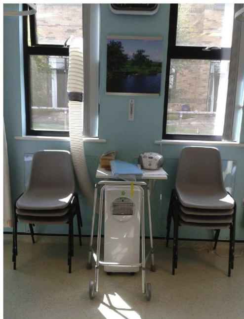
Fig. 21. Portable air conditioning unit, with makeshift safety barriers in a multi-bed room MB2 of Ward 30 during the summer of 2013.
