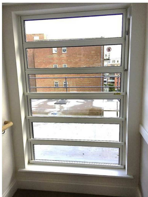
Fig. 22. A secure, safe, well-insulating window ventilation system located at the end of an otherwise blind corridor.
