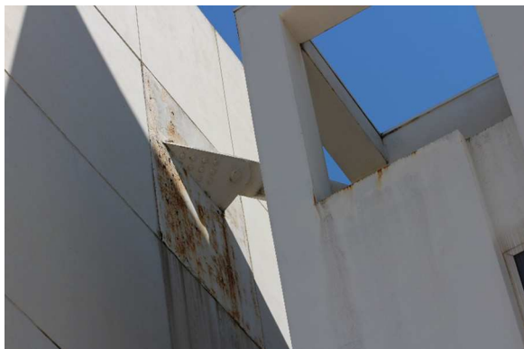
Fig. 15 Presence of rust on the pinned joint of the roof beam (Picture by the author, taken 22/05/2016).
