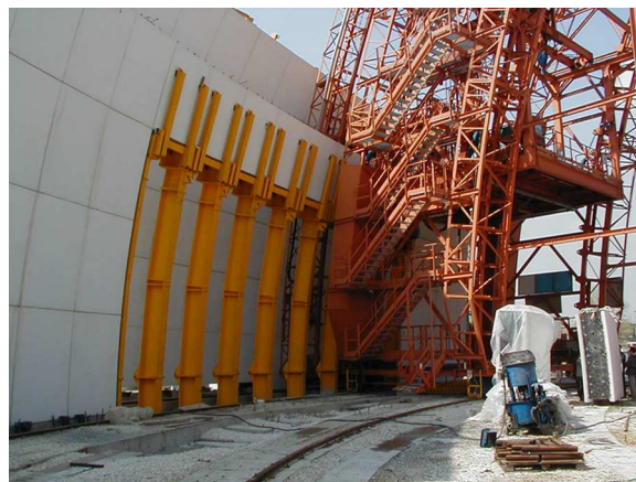
Fig. 3 The travelling crane built to assemble the ashlar of the three shell. (Picture by the author, taken 04/04/2001).
