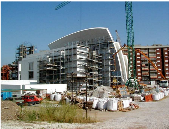
Fig. 5 The northern façade of the parish house during its construction. The shells are completed and the travelling-crane disassembled (Picture by the author, taken 26/06/2012).
