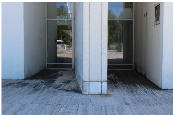
Fig. 7 The area of the external pavement most affected by the acid rain deposits (Picture by the author, taken 22/05/2016).
