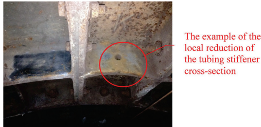
Fig. 2. The example of local reduction in the cross-section area of an underground tubing stiffener.
