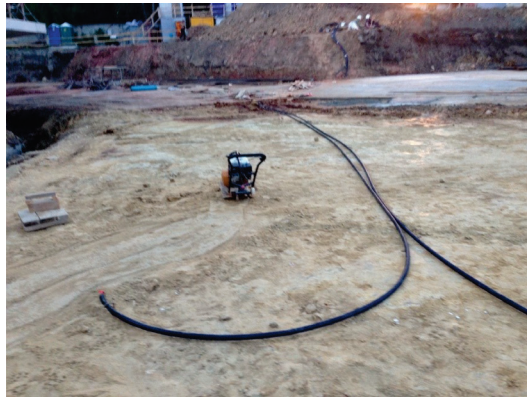
Fig. 5. Overall view of the installation site of pressure gauges.
