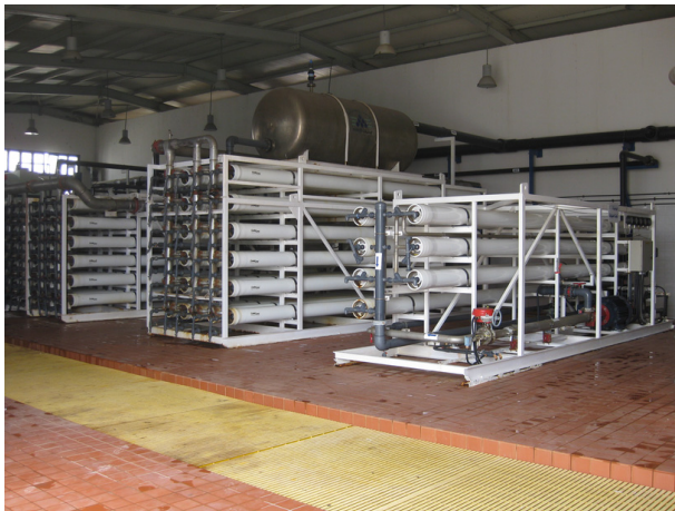
Figure 8. Dahab RO Membrane Unit
