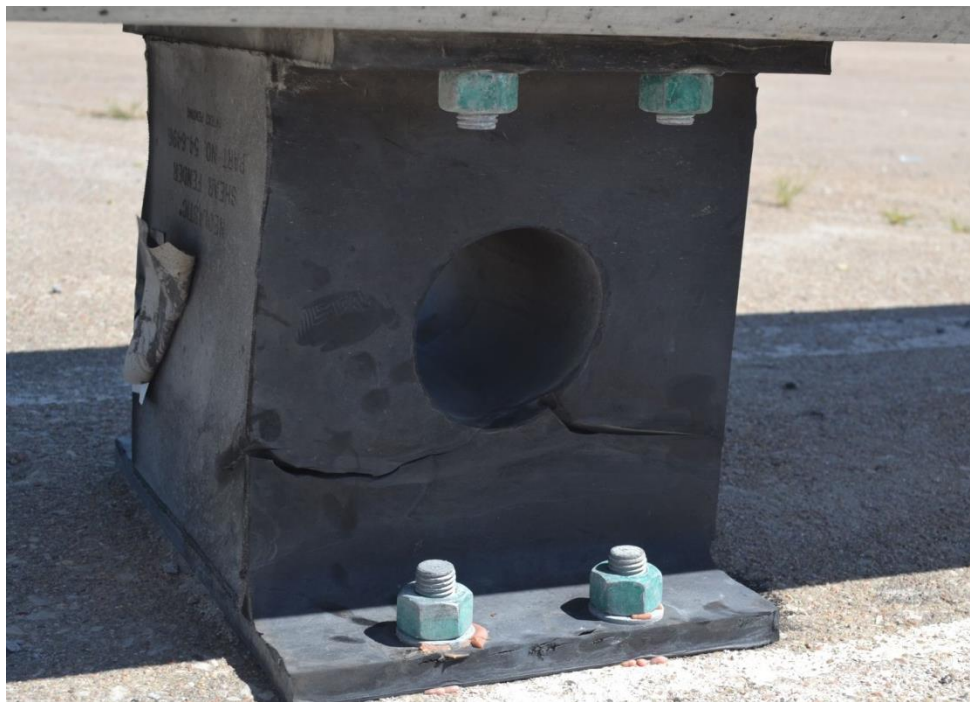
Elastomer Post Damage
