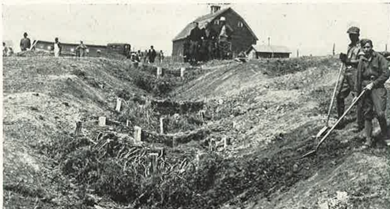
FIGURE 8.—Gully control on the Plum Creek Project. Note the small dams, and that the shoulders of the gully have been shovelled off. This work was done by CCC boys.
