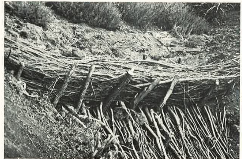
FIGURE 7.—Brush dam in a deep ravine on the Plum Creek Project; view from the downside. Photo by Richard Hufnagle.
