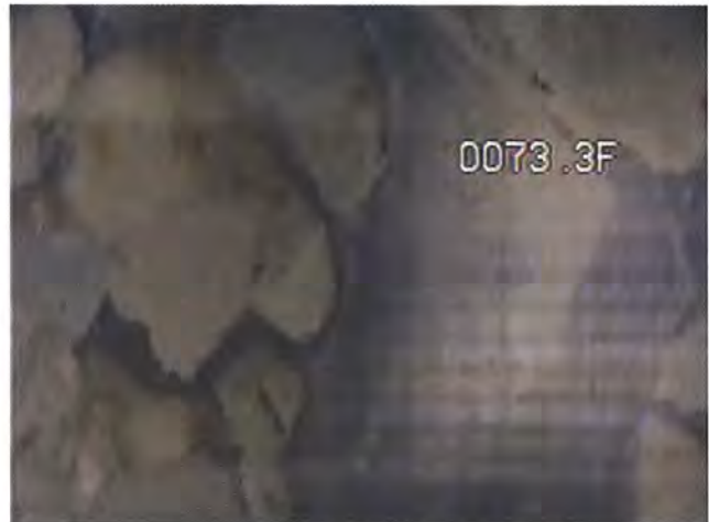
Figure 23. Failure of bentonite chip seal caused by cement grout.
