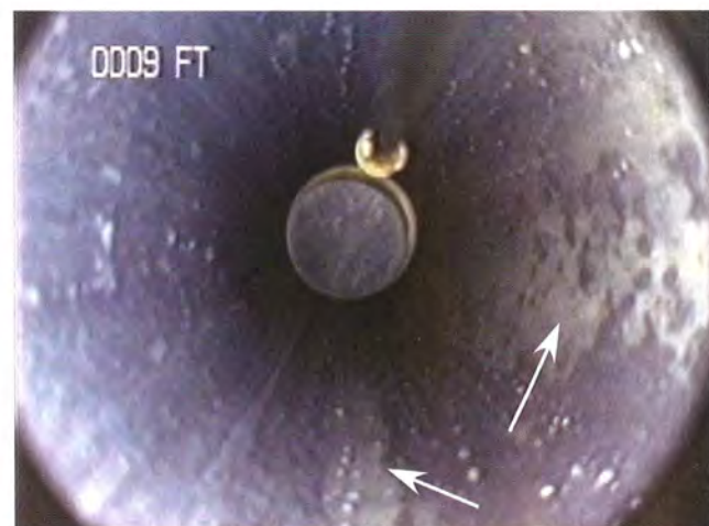
Figure 30. Neat cement appears detached from casing.
