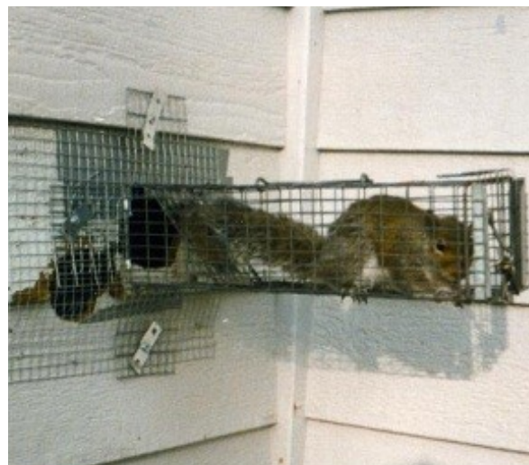
Figure 1. Squirrels can damage homes and other structures. This squirrel has been captured in a live trap near the damaged site.
