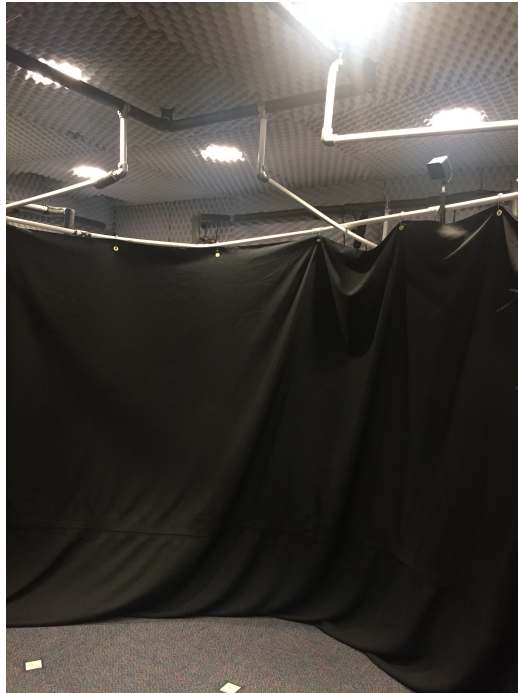
Figure 3.4: Installed acoustically transparent curtain
