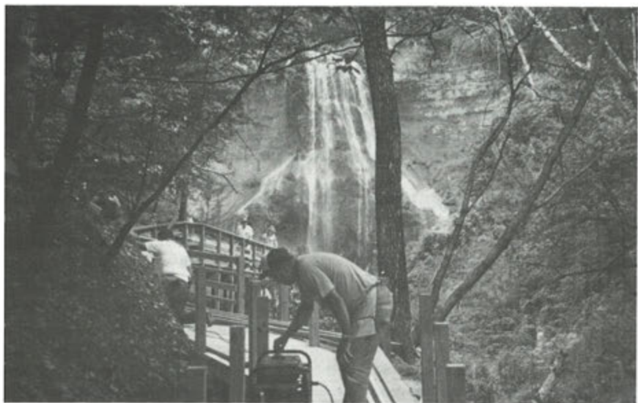
Caspar Yost Chapter of Telephone Pioneers of America built walkway at Smith Falls State Park.
