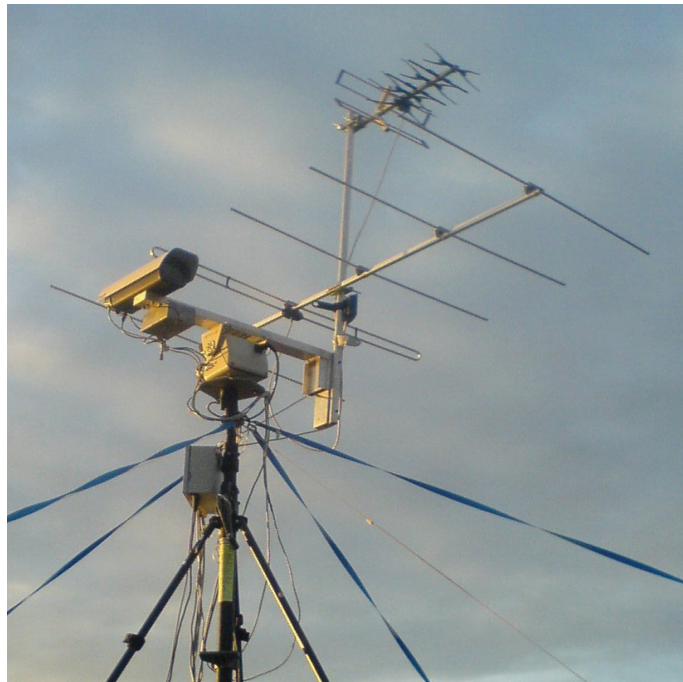
(b) Surveillance channel, DVB-T antenna; Funke Digital TV FFA4522 21/69 [129] (upper antenna), FM radio; TRIAX 5 element [127] (lower antenna).
