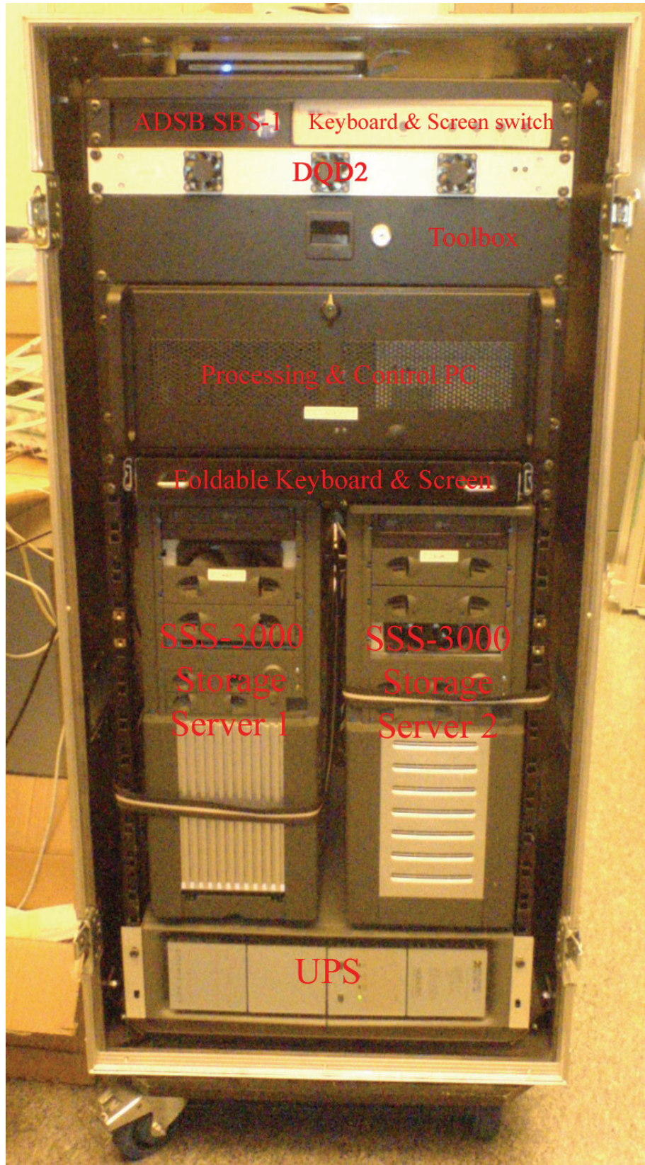
Figure 4.4: The data recording system mounted in a rack.
