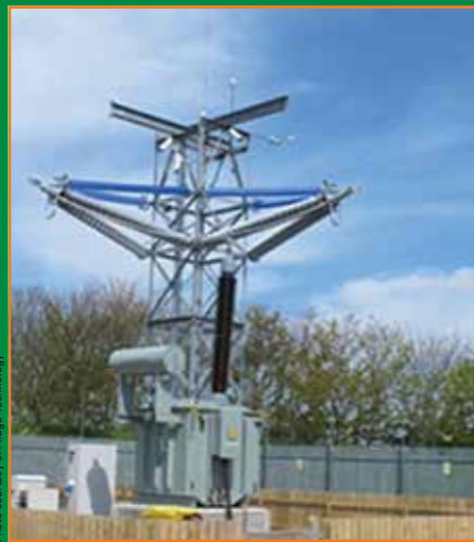
Fig. 11: 400 kV test site.
