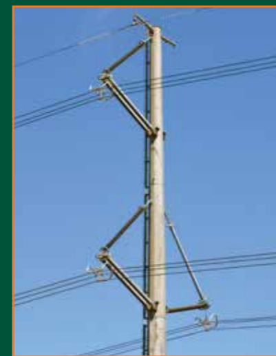
Fig. 5: 420 kV compact line near Cape Town (braced twin post design).
