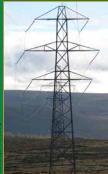
Fig. 2: Example of 'blow out' on exposed 132 kV tower in U.K.
