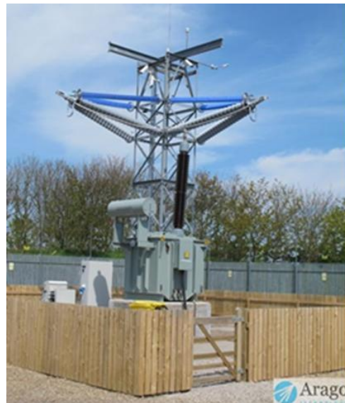
Figure 6 The live test site: fully instrumented and energized to 400 kV system voltages.
