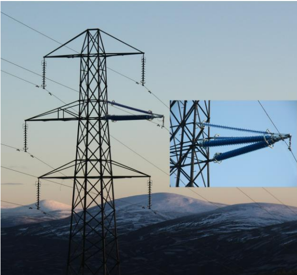
Figure 5 Insulation cross-arm installed on a redundant line in Scotland for two years' load testing.
