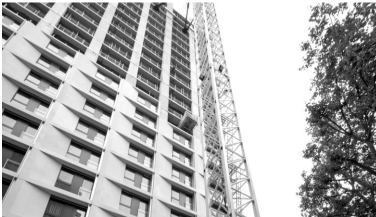
Figure 2: The recently-built Two Fifty One project in London (photo by courtesy of Laing O'Rourke plc)
